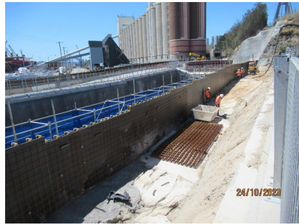
Figure 3.8 The Bays: FRP for construction of the edge of the station box
