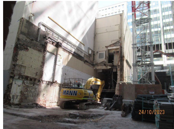
Figure 3.6 Hunter West: Ongoing soft strip; segregation and load out of wastes in the various buildings
