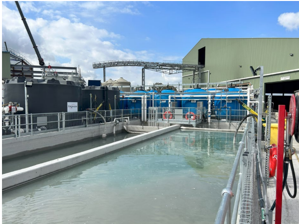
Figure 2.7: Rosehill Site – Water Treatment Plant
