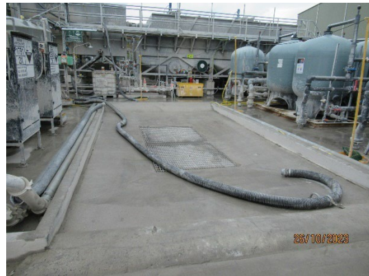
Figure 1 2 Water Treatment Plant (The Bays).
