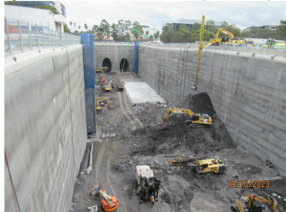
Figure 1.8 Load out of spoil from the Station Box (SOP). Construction of nozzles and blinding concrete in the western end.
