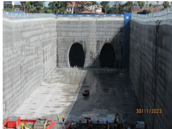
Figure 1.8 Handover has occurred for the Western end of the Station box including the Nozzles (SOP).
