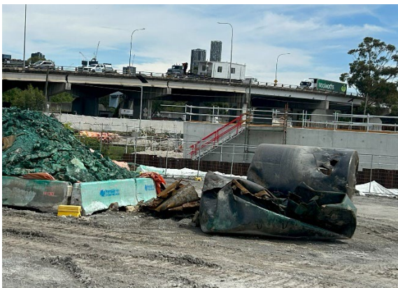
Figure 2.11: Clyde MSF Site – Unexpected Petroleum Storage Tanks removed at 2 Kay Street
