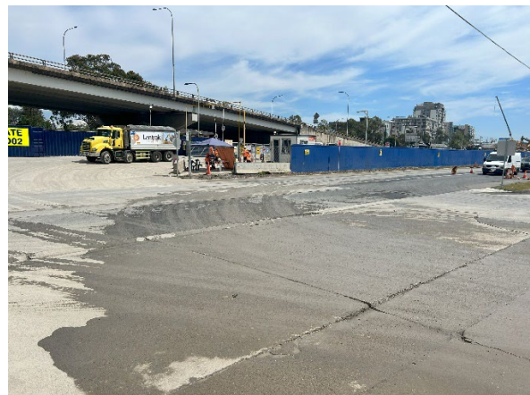
Figure 2.12: Clyde MSF Site – Mud tracking onto Unwin Street prior to clean up
