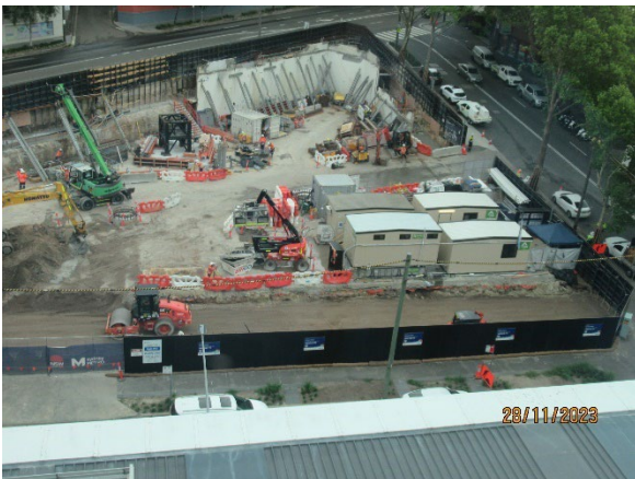
Figure 3.1 Pyrmont East: Tower Crane base installed. Piling pad along Union Street under construction.
