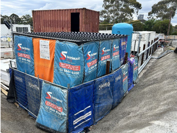
Figure 2.1: Westmead Site –air compressor with additional mitigation measures
