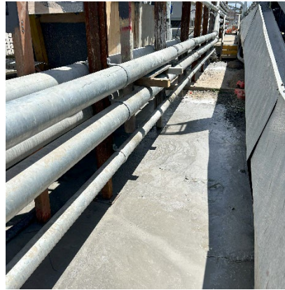
Figure 2.10: Rosehill Site – Grout Plant spill
