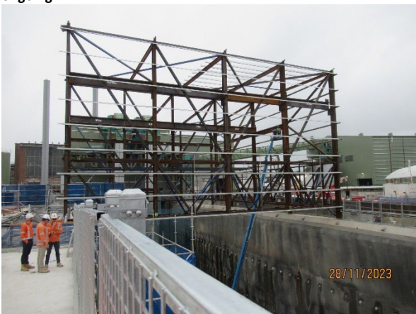
Figure 3.7 The Bays: Frame being constructed for the Segment Shed over the station box
