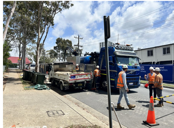
Figure 4.2 Westmead Utility Works: Utility investigations with Vac Truck with truck partially blocking driveway
