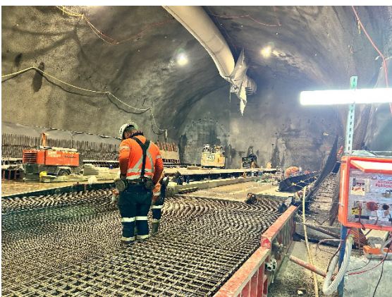
Figure 1 5 Concrete FRP works in the base of the Central Cavern (Five Dock).
