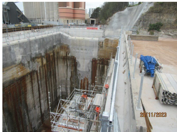
Figure 3.8 The Bays: FRP for construction of the edge of the station box near completed
