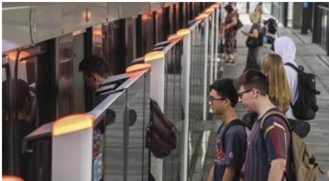
Image: North West safety doors.
