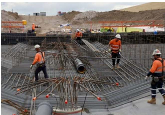
Image: Establishment of site at the Sydney Metro Western Sydney Airport project.
