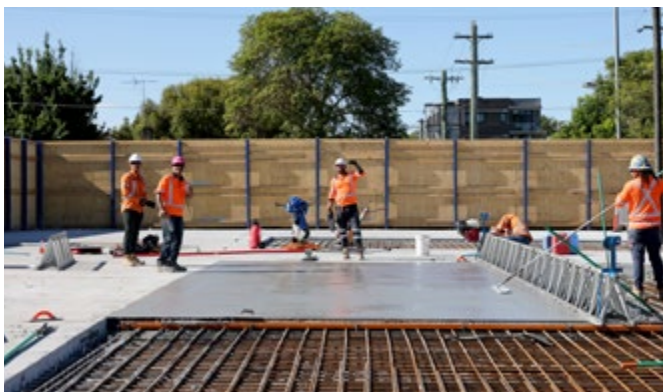
Image: Concrete works at the site of Sydney Metro's station at St Marys.
