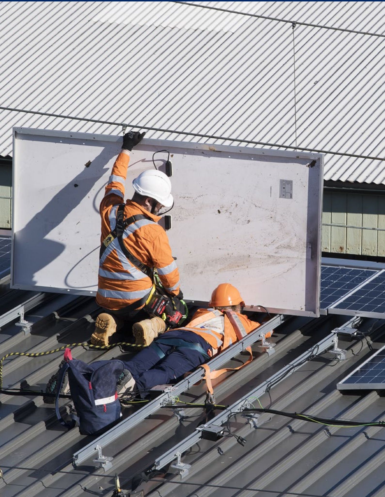
Image: Solar panels are being installed as part of Sydney Metro's major upgrade of Central Station.
