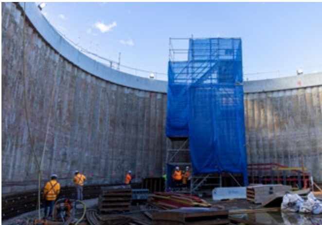
Image: Work continues on the station box and service shaft at Sydney Metro's new Airport Terminal Station.
