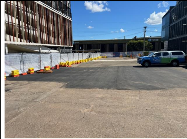
Hot mix has been applied to the disturbed area within the compound.
