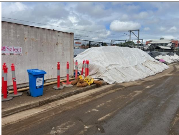
Excavated material has been stockpiled and covered in geofabric prior to removal.
