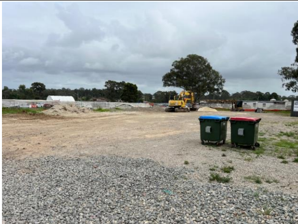
The compound has been demobilised with only a few materials left to load out.
