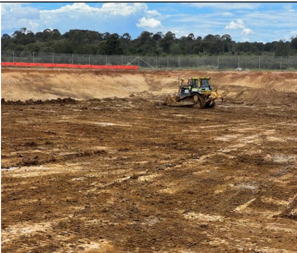
Cosgroves Creek: Works continue in the biofiltration basin, with material being excavated.
