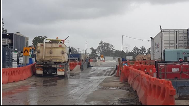
Orchard Hills view north: Wheel wash now followed by concrete runway and manual wash.
