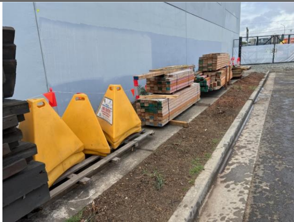
Materials are stored on the footpath adjacent to the newly planted garden bed. LoR to make submission to SM and TfNSW regarding usage and potential rehabilitation
