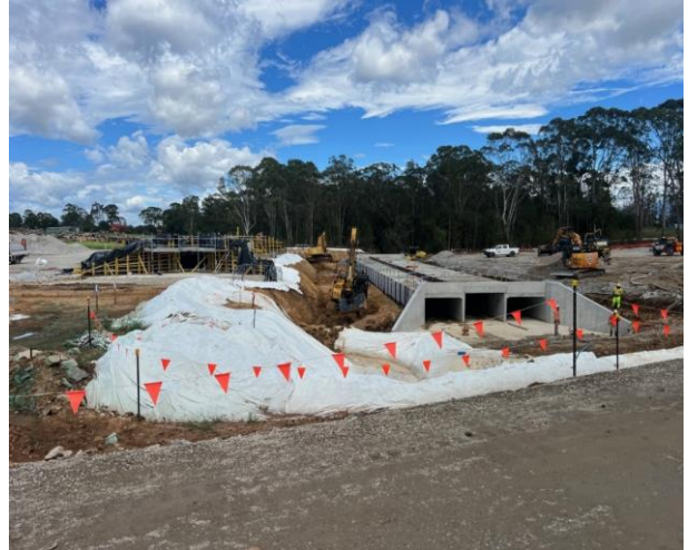
Unnamed tributary culvert and fauna crossing: Works progress to a high level of environmental compliance.
