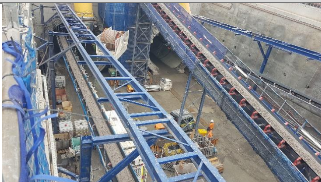
Orchard Hills view North: Portal activities, with TBM spoil conveyor delivery to the surface.
