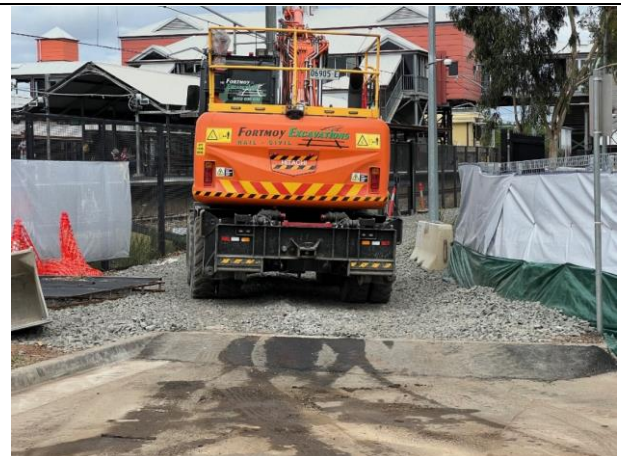
Ballast has been applied to the area where machinery will be parked.
