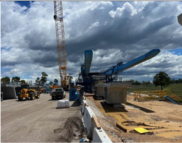
Luddenham South: Viaduct works crossed Luddenham Road and continue towards Cosgroves Creek.
