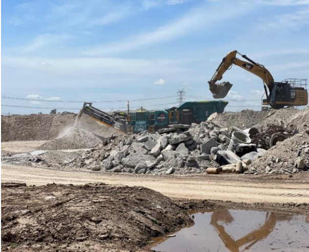
PS105: Rock crusher has been set up behind bunds and with water sprays to limit dust migrating from the site.
