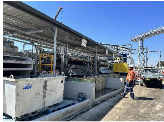
Figure 2.10: Rosehill Site – 50L/s Water Treatment Plant operating
