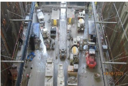
Figure 1 1 Base of the station box showing various plant operating (The Bays) and TBM support activities.
