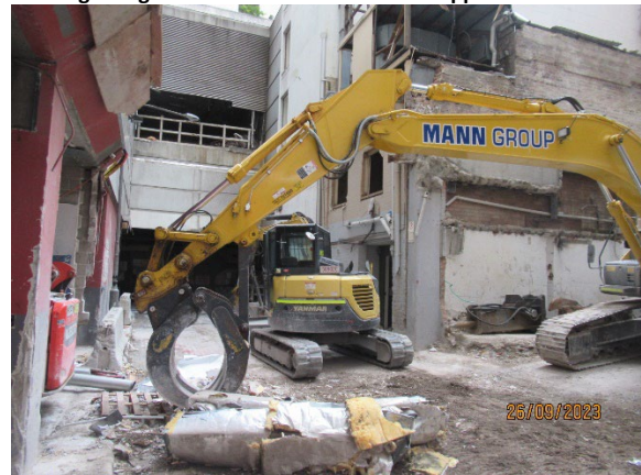
Figure 3.6 Hunter Street West: Ongoing soft strip; segregation and load out of wastes in the various buildings
