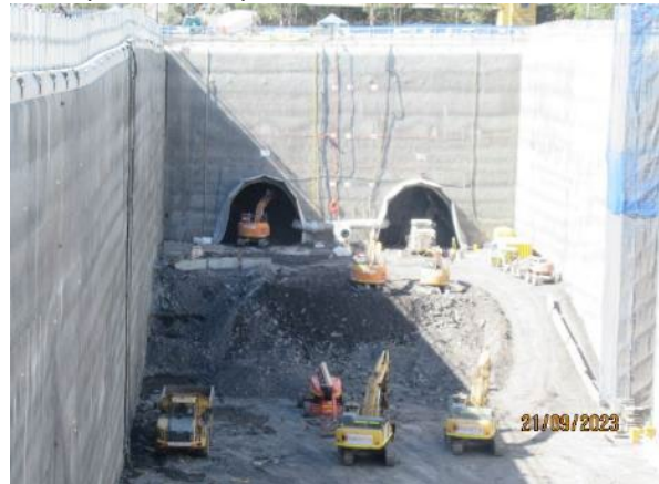
Figure 1.8 Excavation of the Station Box (SOP). Construction of nozzles in the eastern end.
