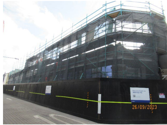
Figure 3.4 Pyrmont St West: Scaffolding installed around the building being removed after demolition of upper floors
