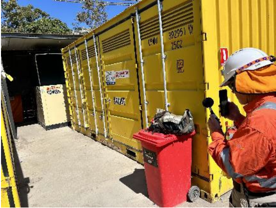
Figure 2.1: Westmead Site –AA monitoring air compressor
