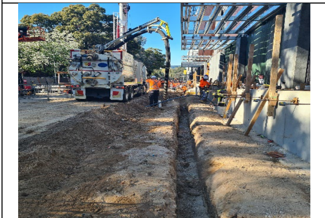
Northern Building end - Cope St Site Compound: NDD in progress for future services and formwork in progress for U shaped garden bed.
