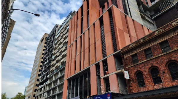
Pitt St South (PSS): glazing work and façade installation (view from Bathurst Street)
