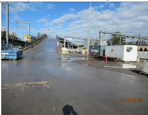
Sydney Yard: Much of the equipment that had been stored in the laydown area has been removed. Use of the area by other contractors.
