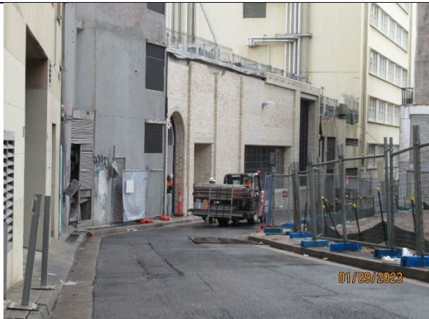
Eastern Entrance: View from Randle Lane. Scaffolding being placed to allow for remedial works on the façade and roof of the building.
