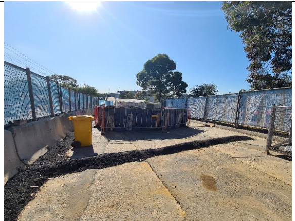
Artarmon BPS: Joint Bay (Carlotta St) reopened on 29/08 and joint replacement underway.
