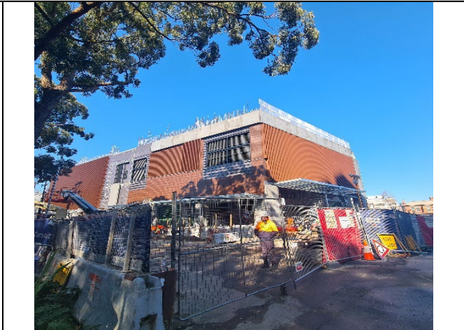
Northern Building (View from Raglan St): Façade installation; fit out and service installation works continuing.
