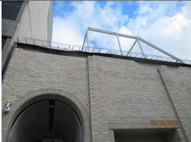
Eastern Entrance: View from Randle Lane with new frame installed on the roof
