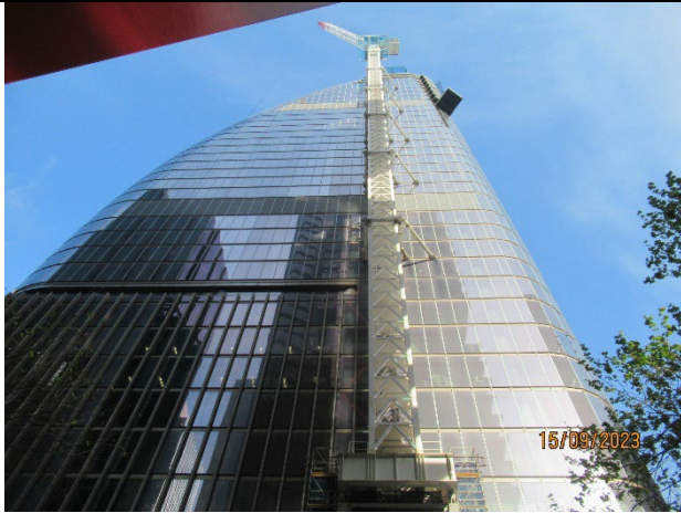
Martin Place North: View from Elizabeth Street near the corner of Hunter Street. Ongoing façade construction. SE Tower crane removed.
