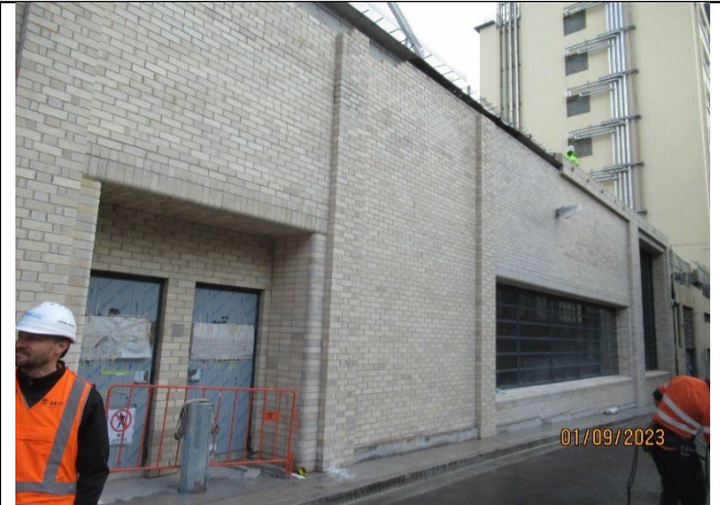
Eastern Entrance: View from Randle Street showing damaged bricks near roof level.
