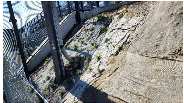
Lakemba – rail embankment landscaping (note section missing plant landscaping raised with Sydney Metro to address with follow-on contractor).
