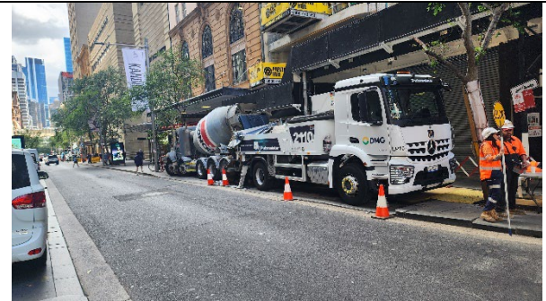
PSN: OSD concrete pump on Castlereagh Street (noting noise mitigation could be better).
