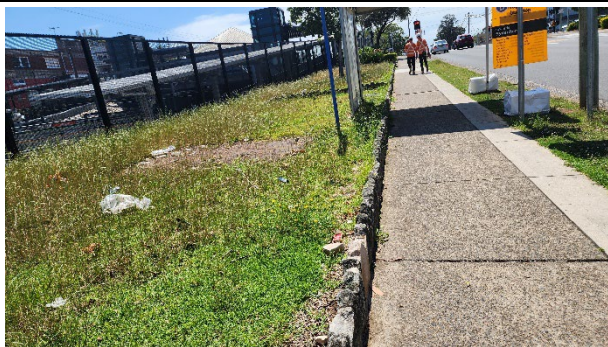
Wiley Park – damage to sandstone edging.
