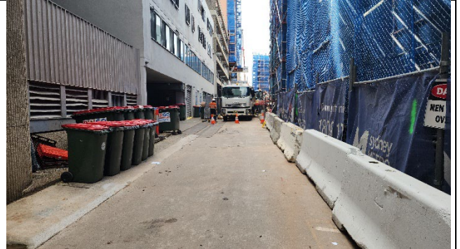
Clark Lane North minor ancillary facility – area was maintained, and no sediment was observed exiting the minor facility. Metro approved banner mesh had been installed.
