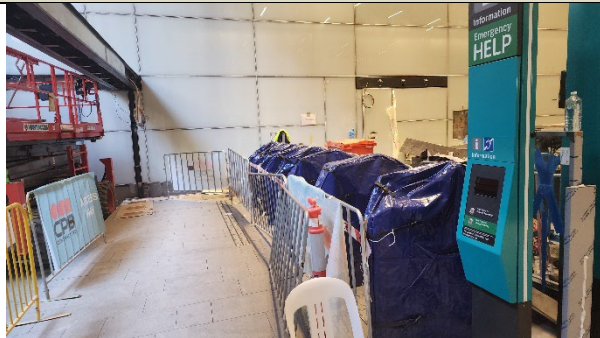
Pitt St South (PSS): Opal card readers installed.
