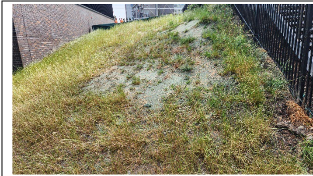
Canterbury – MSB hydroseed stabilisation of batter (note patch due to shallow rock).
