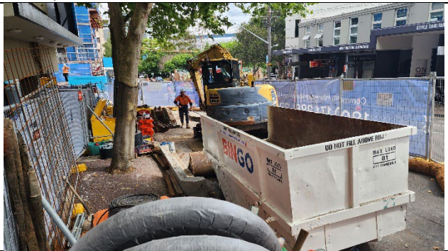
Clark Street Public Domain works (trenching) – Erosion and sediment control installed and good tree protection.
