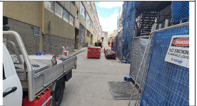
Clark Lane South – Traffic control is in place and erosion and sediment controls maintained.
