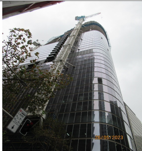
Martin Place North: View from street level on Elizabeth Street. Tower crane in operation
