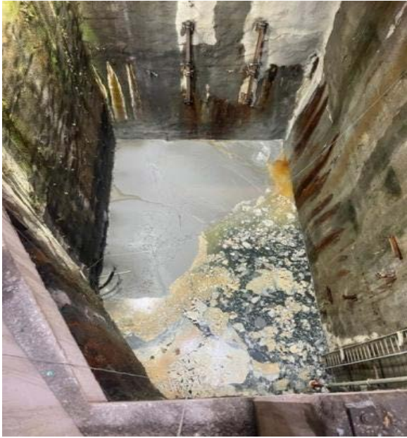
Backfill of the northern shaft (groundwater seepage and bleed water on top layer)
