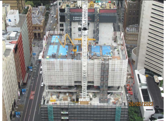
Martin Place South: View from north tower. Concrete works for floor slabs being undertaken
