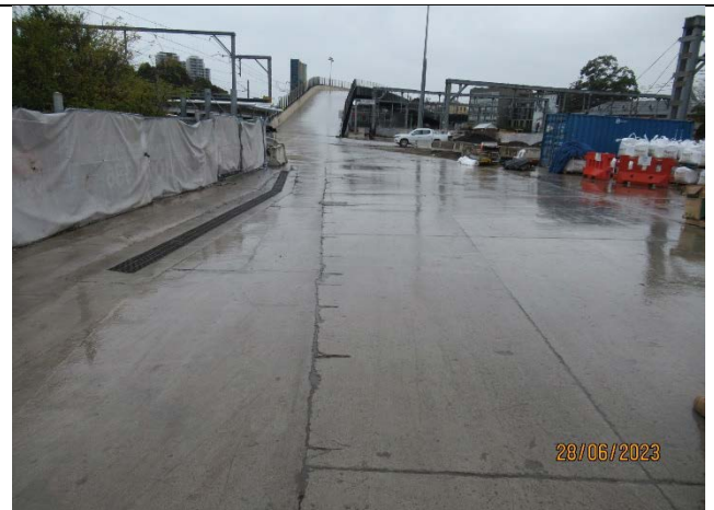
Sydney Yard: Reduced plant and equipment stored in the area. Shared usage by various contractors
