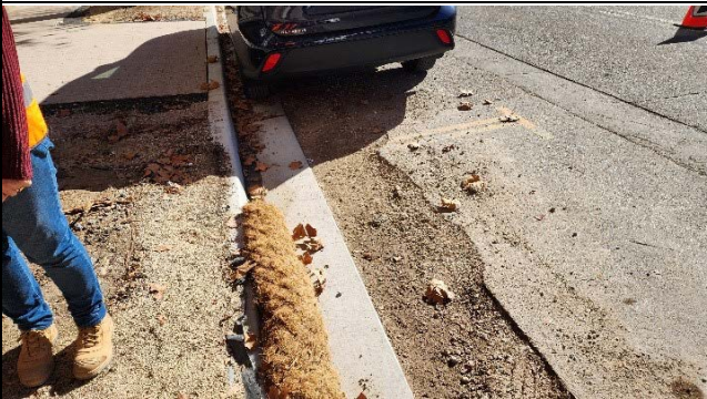
Clark Street – potential ERSED risk from traffic driving over DGB
