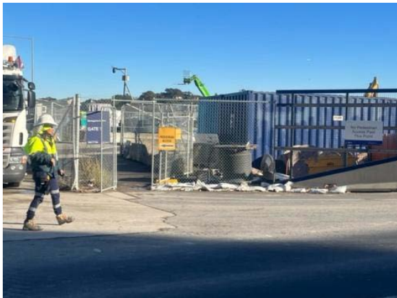
Signage at Hickson Road site access to be reviewed
