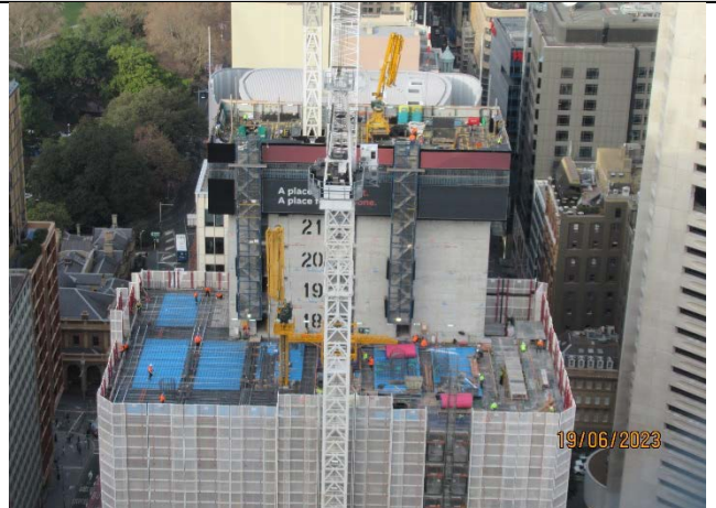
Martin Place South: View from north tower. Concrete works for floor slabs being undertaken
