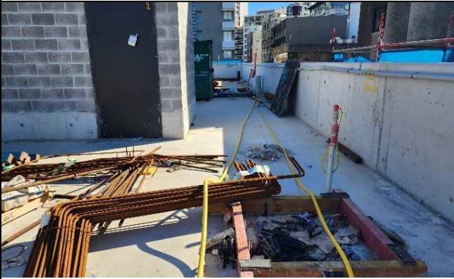
Site A Level 2 noted minor rubbish required removal
