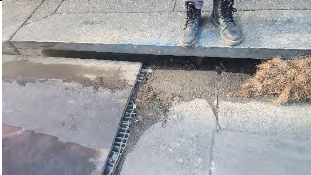
Clark Lane South – maintenance of ESC required
