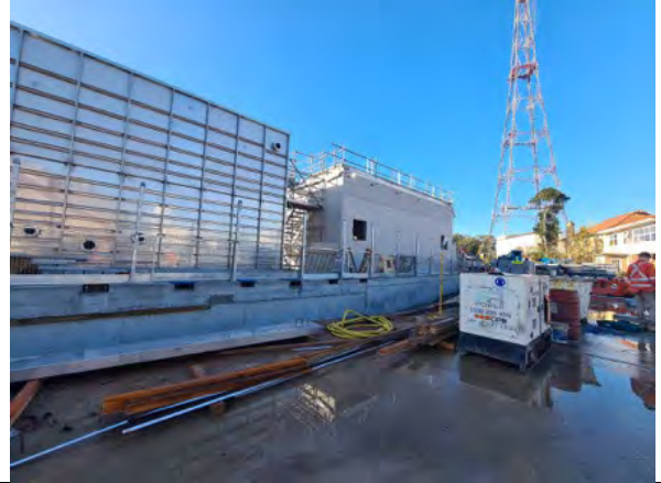
CDS: Structural steel install/cladding works underway for fire pump room and tank storages.
