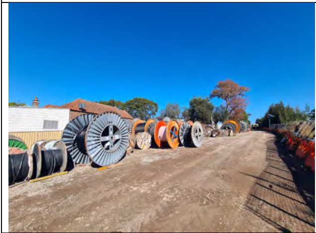
Belmore St Site Compound and Laydown: Cable storage and surrounding area observed to be generally tidy.
