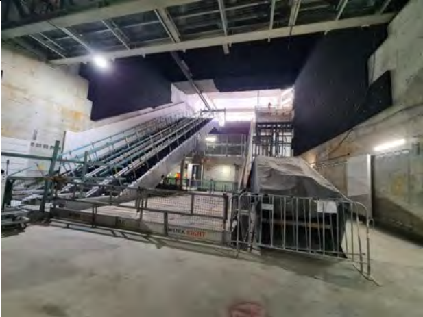
VCS: Preparatory works for escalator install underway for future split access onto Miller St and Denison St.
