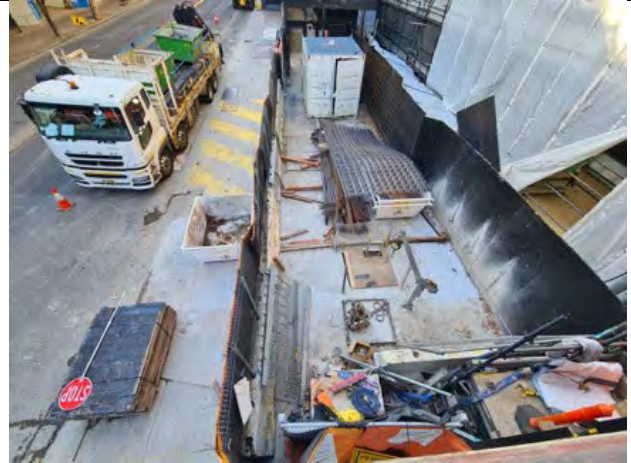
VCS Miller St Stormwater worksite: Stormwater works on Miller St within the footpath completed.
