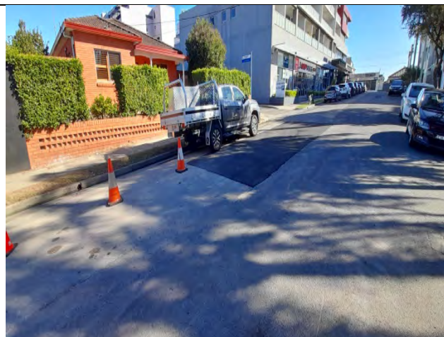
Cooks Ave Joint Bay: Cooks Ave Joint Bay worksite works are noted to be completed. Note construction cones are related to the site adjacent to Cooks Ave Joint Bay
