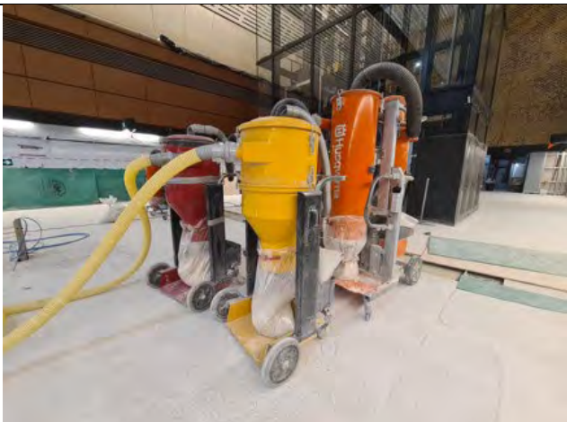
Station Cavern: Platform tiling and grinding works underway; with dust from tile grinding captured
