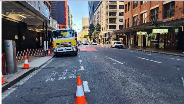
Pitt St South (PSS): Bathurst Street noting road plates for utility works
