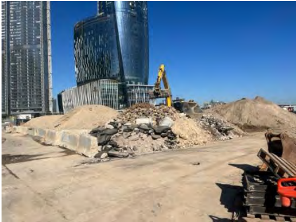
Stockpiling in the main laydown area – stockpiles not in use to be covered
