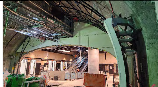
PSS Adit sandstone archway entrance to southern escalators and sandstone wall installation
