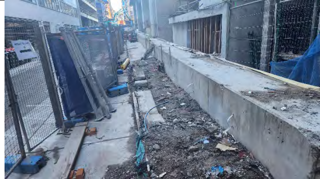
Capping Beam removal – noting ESC required for exposed areas to prevent sediment runoff from site
