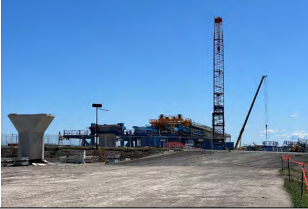
Luddenham North - The bridge gantry rotated to commence working towards Cosgrove's Creek
