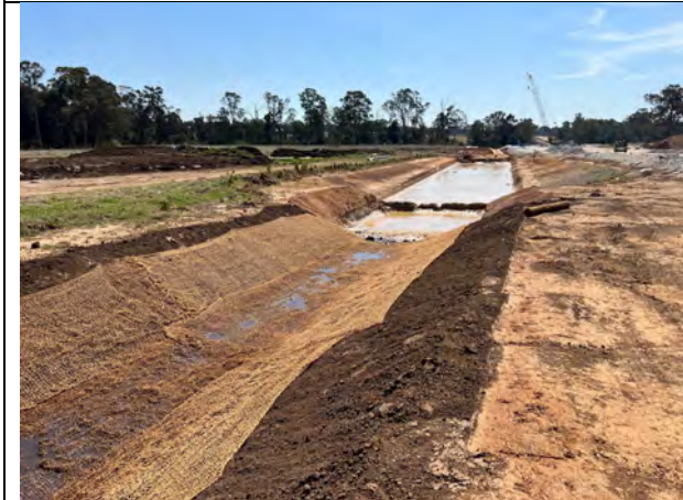
Blaxland Creek - The forebay of the basin at Blaxland's Creek reduces sediment load on the main basin.
