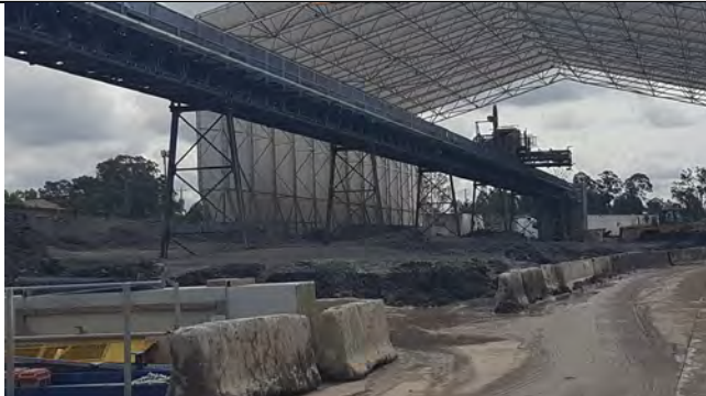
Orchard Hills view north from station box: TBM Spoil delivery conveyor and storage area
