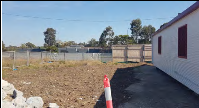
Claremont Meadows: Mulch use as control & CPB improving installation of western sediment fence.
