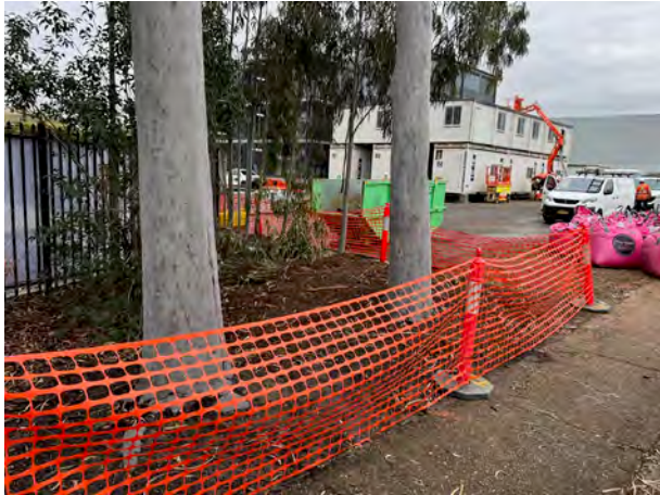
Site compound - TPZ placed around trees to be cleared, until ecologist confirms hollows are clear.
