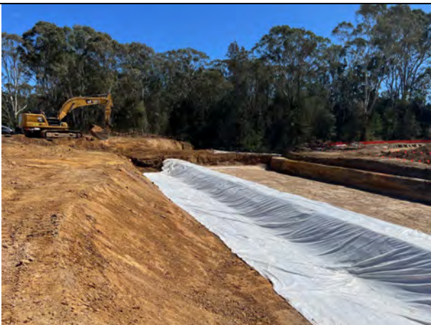
Orchard Hills - Floor of unnamed tributary west of Blaxland Crk excavated ahead of the blinding slab pour
