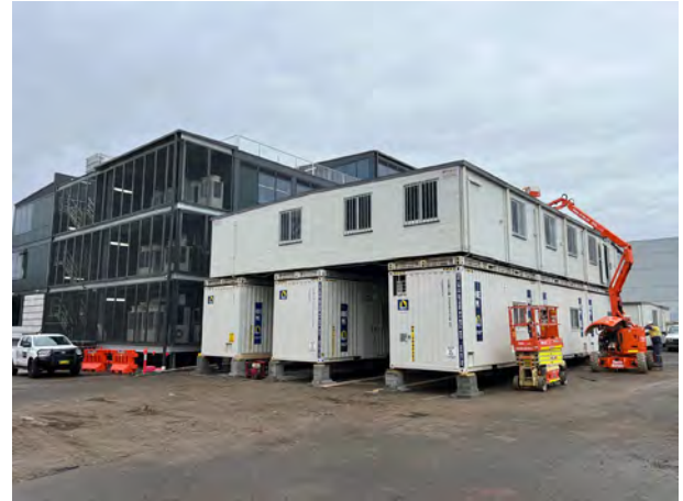
Site compound - Site compound establishment had approximately another six weeks to go
