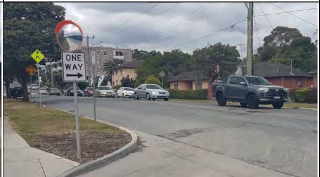
St Marys Philip St: View southeast of area of asphalt to be repaired .
