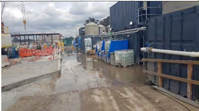
Orchard hills view south: General housekeeping required in the water treatment plant bund.
