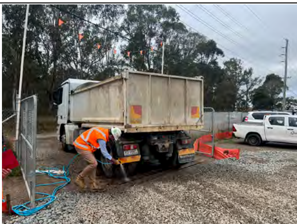
Gipps St Site compound – manual wheel washing was employed during wet conditions
