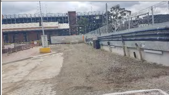
St Marys – Area and controls stable and tidy in northwest areas near goods shed.
