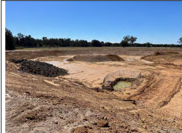
Cosgrove's Creek - The flood retention basin is almost dry, once it is work will recommence on it
