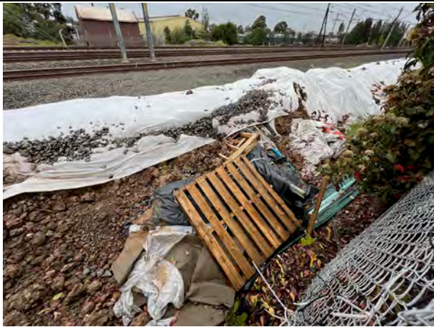
Rail corridor - Geofabric in the back of this spoil stockpile to be extended to cover all exposed faces, and rubbish to be removed into designated skips
