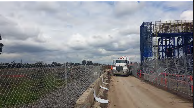
Orchard Hills - View south of Installation of ErSed controls at interface of SSTOM and SBT sites.
