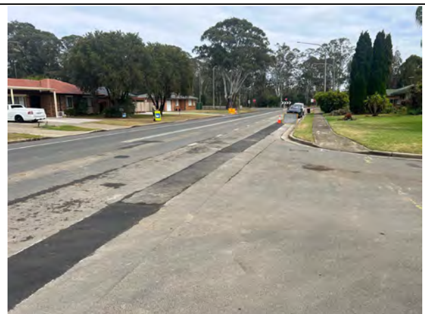
Solander Drive to Mamre Rd- Works progressing well with no complaints received from residents
