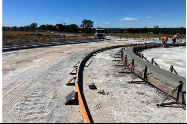
Luddenham North - Roundabout kerb poured, and Out of Hours works are due to commence
