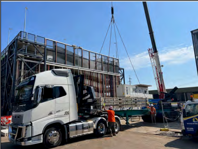
SPO - Site offices are being dismantled and handover is expected to occur on 15/09/23
