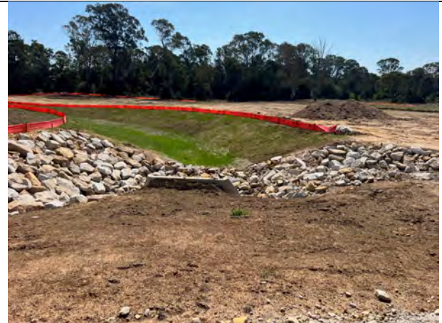
PS105 Stockpile - Rock lining, hydromulching and jute matting used to stabilise drainage lines effectively
