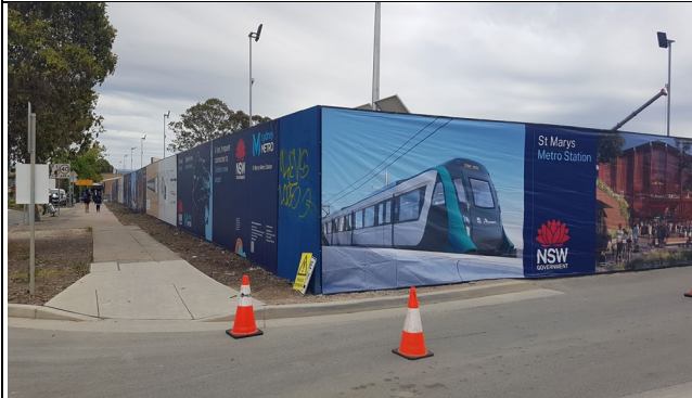
St Marys – Installation of SM WSA graphics on north west corner of Phillip St. and Blair Av..
