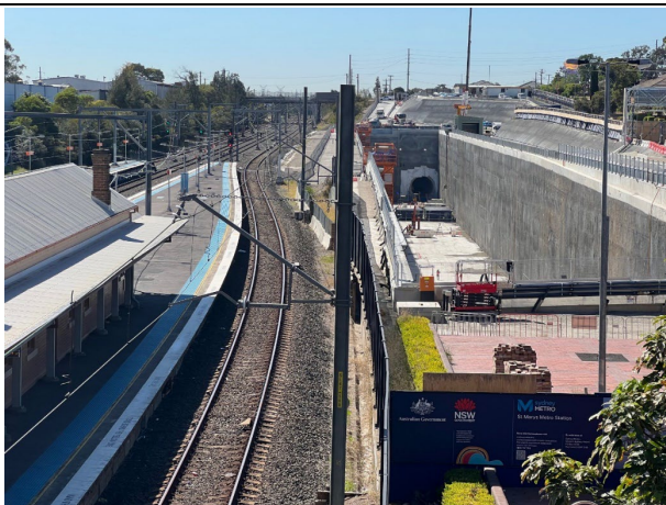
A view of the of the platform where the SBT rock anchor / FSM pile interference could occur
