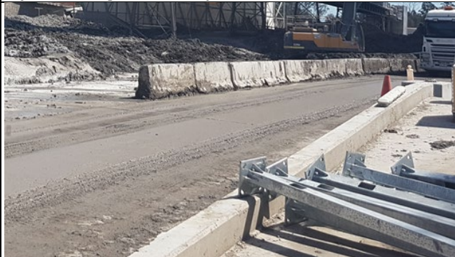
Orchard Hills view northwest – Condition of internal haulage road required improvement.
