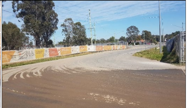
Claremont Meadows: Tracking noted from southern site access onto Gipps Road.
