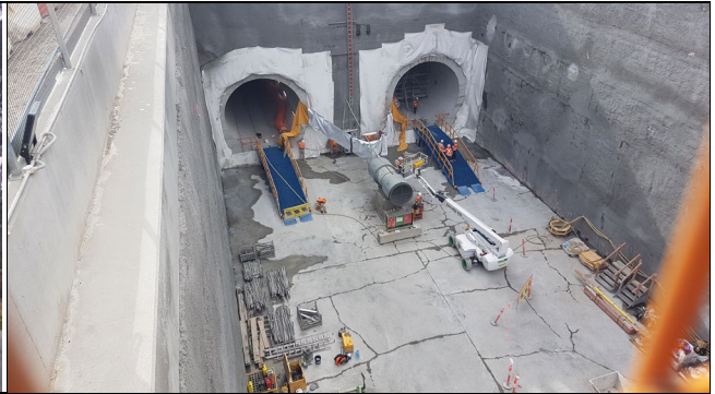
St Marys: View east of station box stub tunnels completed, with extraction fan to remain.
