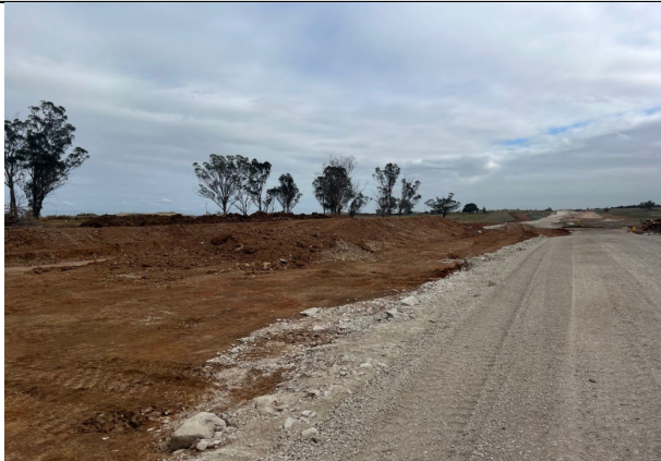
Sandstone has been placed on the formation adjacent to the EDR compound
