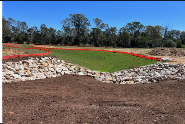
The rehabilitation at PS105 has been successful and has reduced the ERSED risk
