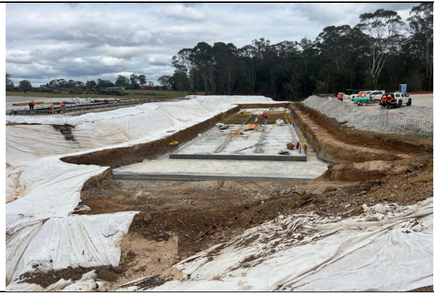
The culvert and fauna crossing at the unnamed tributary are being constructed to a high level of environmental compliance
