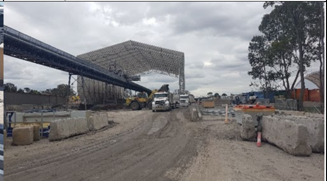
Orchard Hills: TBM Spoil storage area condition and management of haulage areas improved.
