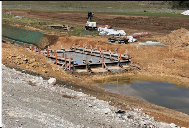
The basin at Blaxlands Creek has been stabilised and is in the process of being made into a bio basin
