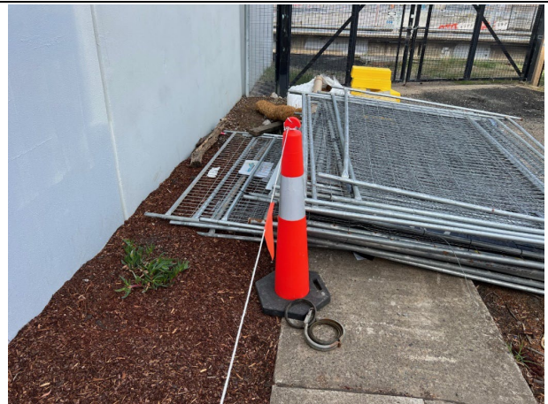
The ATF stored on the mulch garden bed needs to be moved and the flagging returned to the end of the garden bed
