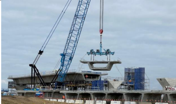
Luddenham Station - Segments of the viaduct continue to be lifted into place following an exact sequence
