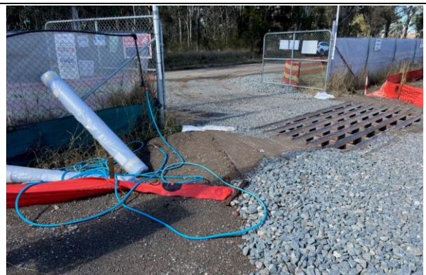
Site compound - The ballast, hose and rumble grid have mitigated mud tracking from the compound
