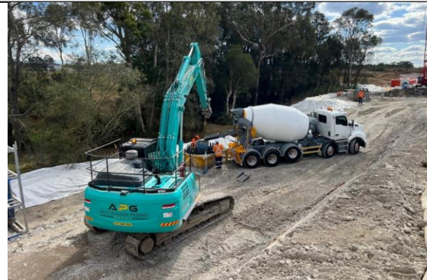
Blaxland’s Creek - Controls have been established to reduce the risk of water pollution during concreting works
