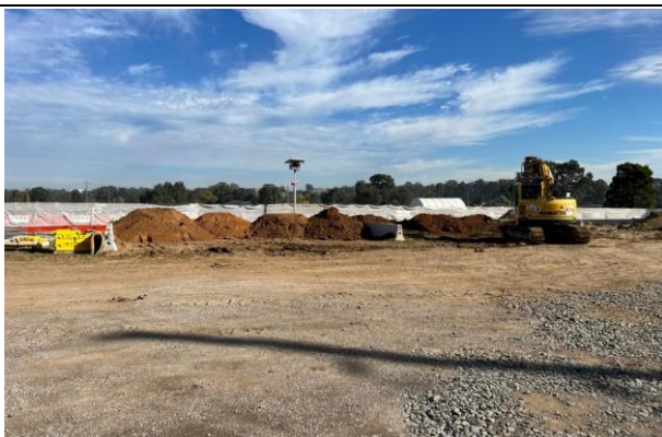
Site compound - The bays in the site compound were neat and tidy with no evidence of cross contamination
