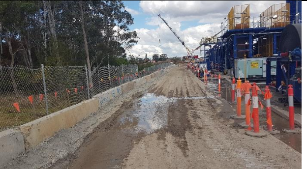
Orchard Hills - View south of concreted eastern haul road with jersey barriers and concrete berm.
