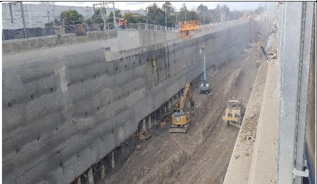
St Marys: view east of station box excavation. Note mist from water misting cannons
