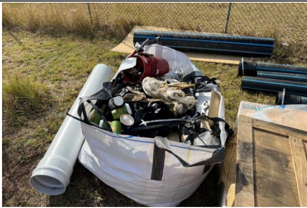
Old Luddenham Rd - Bulka bags are being reused as mobile bins across alignment. Good practice.
