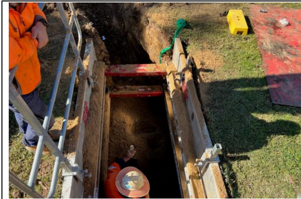
Mamre Rd - The first bore underneath Mamre Rd is complete and was in the process of being backfilled
