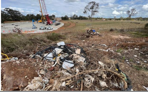
Blaxland's Creek - Unexpected landfill material has been found north of Blaxland's Creek.
