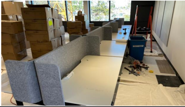
SPO - Internal fit out has progressed and installation of work spaces is nearing completion
