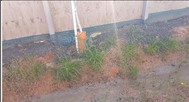
Bringelly: Northern swale requires desilting and trimming and sediment fence requires repairs.
