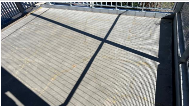
FSM - The landing on the station stairs has cracks and needs to be scabbled in the upcoming OOHW
