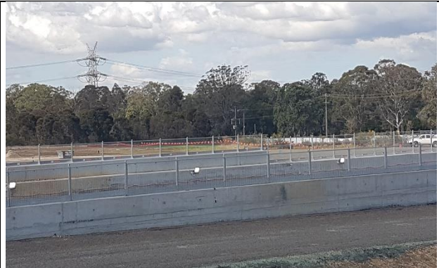
View to Lansdowne Rd.– Areas north of road stabilised and ready for handover to SSTOM.
