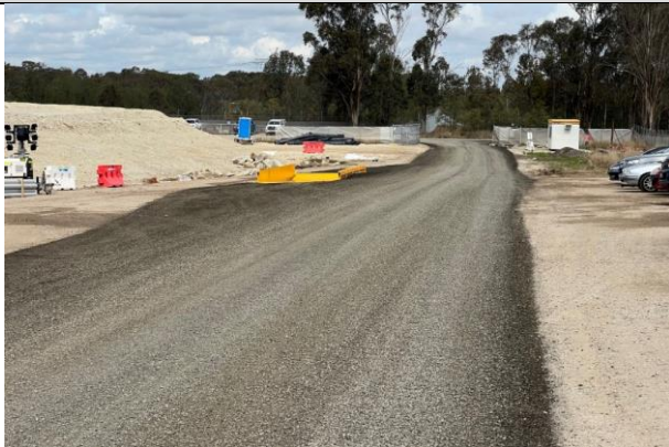
Patons Lane - The wheel wash and chipseal at Patons lane has been installed
