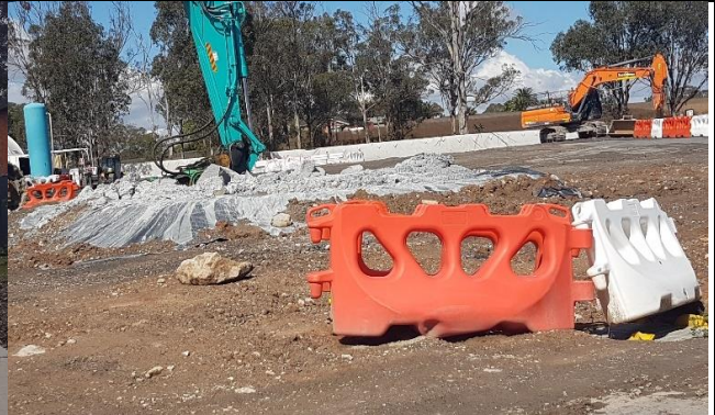
Bringelly: Concrete washout overtopping with cured surplus concrete
