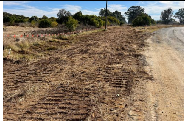
Old Luddenham Rd – Pipe trench at Old Luddenham Rd backfilled and topped with original topsoil.
