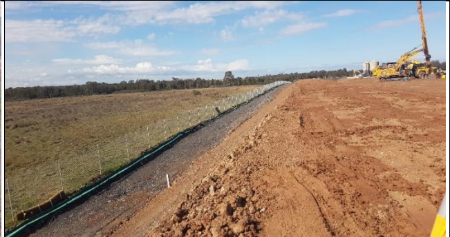
Aerotropolis: Eastern dirty water swale, top and batter of embankment require stabilisation.
