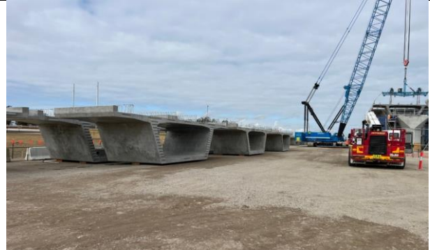
Luddenham Station - The viaduct segments are stored in an exact sequence ready for lifting into place
