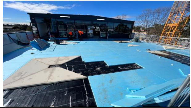
SPO - Works on the top floor continue with this foam flooring layer being installed
