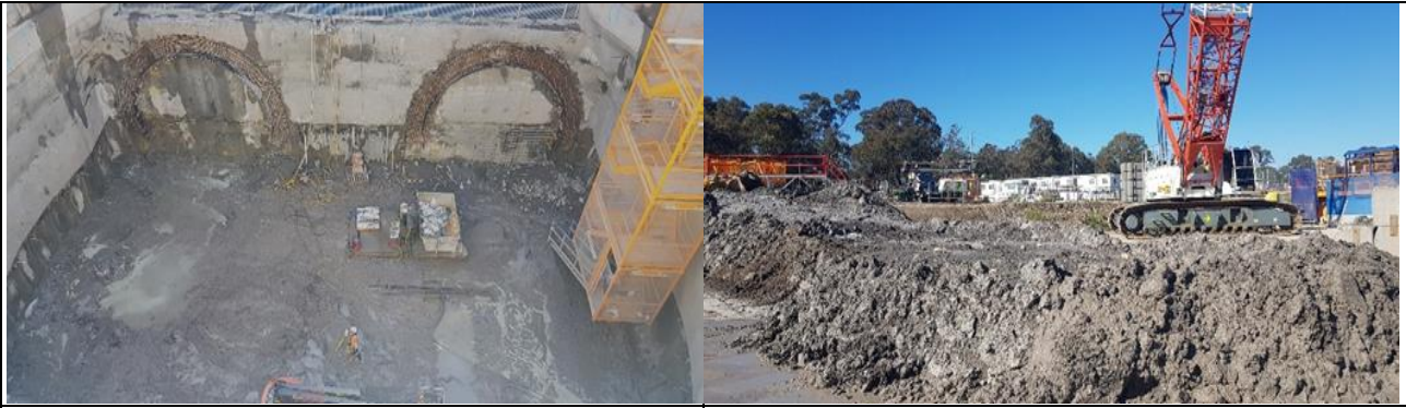
Claremont Meadows: Shaft Excavation within 2 m of completion. Claremont Meadows: View south east from north west corner with spoil bin in foreground
