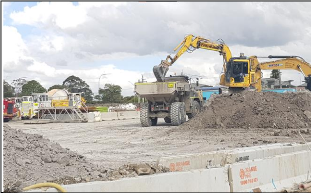
View south east along Gidley St.: Height of spoil stockpiles reduce below hoarding.
