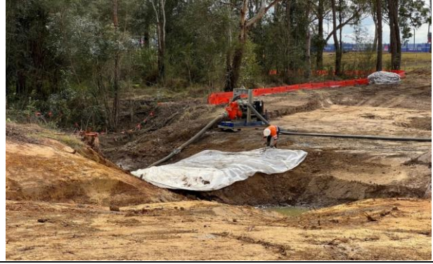
Unnamed tributary - The pump around installed at the unnamed tributary to divert SBT discharge from culvert
