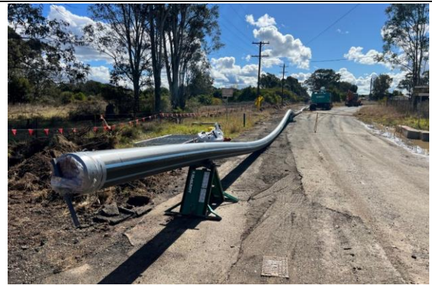
Old Luddenham Rd - Pipe has been joined and ready to be installed in the ground, but delayed by recent rain
