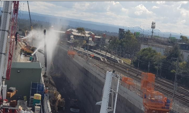
St Marys: view west of station box excavation. Note mist from water misting cannons
