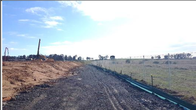
Aerotropolis view north: eastern boundary silt fence requires keying-in, and tensioning.
