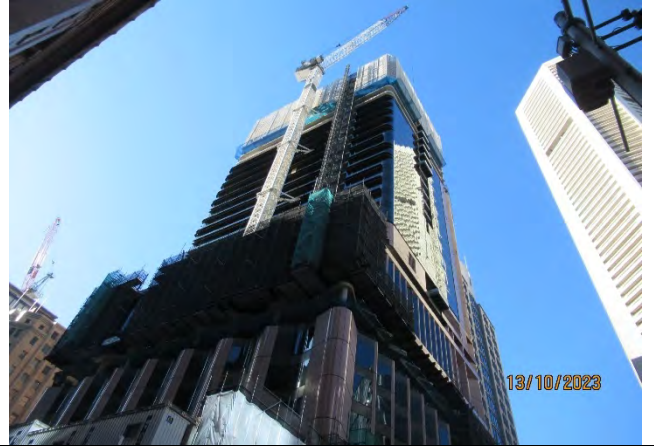
Martin Place South: View from Martin Place west of Castlereagh Street. Concrete pumping from Castlereagh Street.
