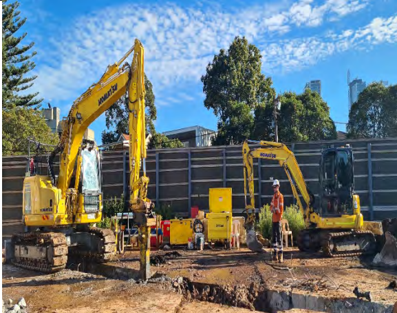
CDS: Trenching (hammering) works for stormwater connection underway. Observed operator wetting down work area during hammering (good practice)
