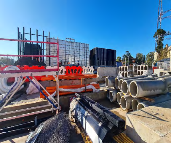
CDS: Installation of pipework and connections in progress for hydrant water tank.
