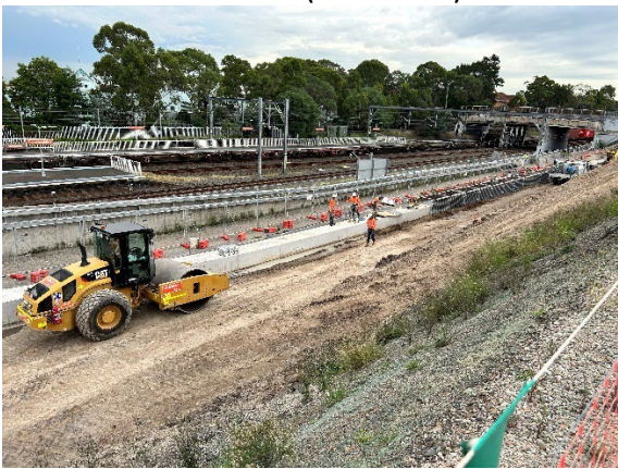
Figure 2-7 Capping beam construction on the lower side of the station box at North Strathfield
