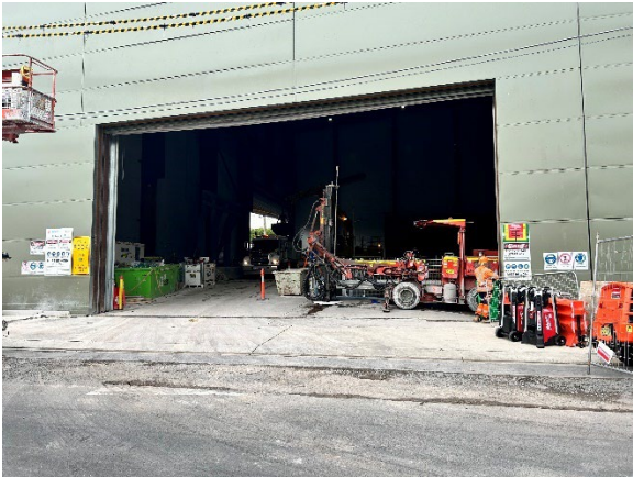
Figure 2-5 Ongoing excavation of the eastern shaft and loading of trucks within the acoustic shed (Five Dock-east).
