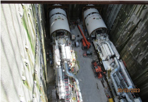
Figure 2 1 Tunnel Boring Machines being assembled in the base of the station box. (The Bays)
