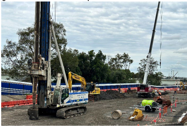
Figure 4.5: Clyde Dive site – Piling for the Dive Structure along the ATC boundary
