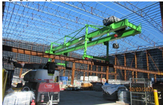
Figure 2 4 Installation of panels for the acoustic shed ongoing. Roof to be installed (Burwood North)
