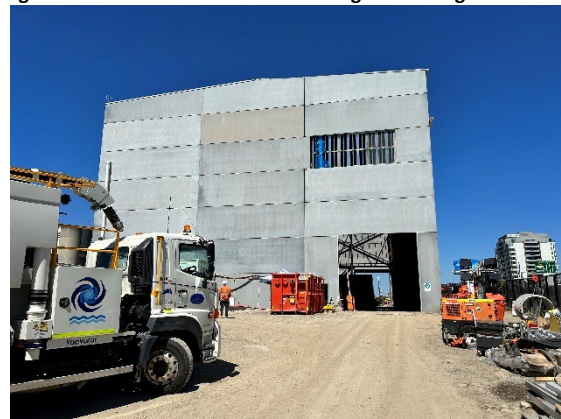
Figure 4.6: Clyde Dive site – Acoustic Shed
