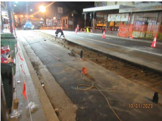
Figure 1 1 Placing steel mesh in the trench after removal of the temporary pavement.
