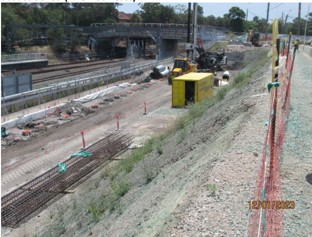
Figure 2-7 Ongoing piling on the lower side of the station box at North Strathfield
