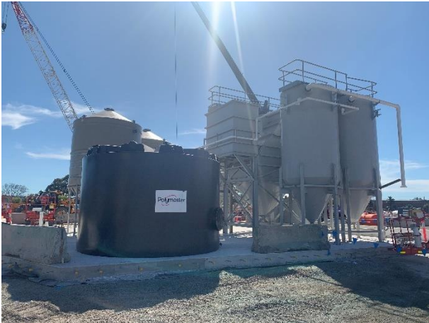
Figure 4.9: Rosehill site – long term water treatment plant assembly
