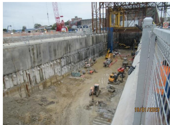
Figure 2 2 Ongoing excavation of the station box (The Bays). Water pumped to the WTP.
