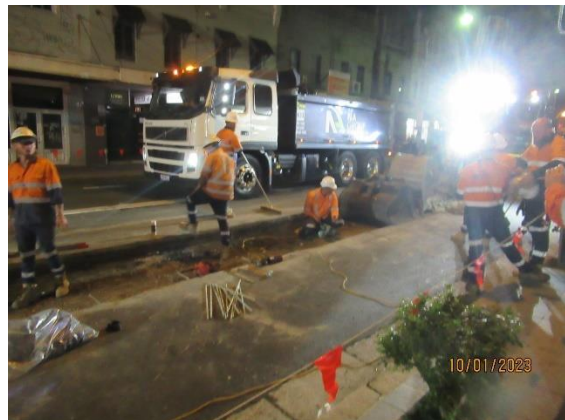
Figure 1 2 Placing steel mesh in the trench after removal of the temporary pavement.
