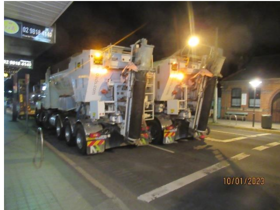
Figure 1 4 Bulk (dry) concrete trucks on site ready to supply concrete for the final pavement.
