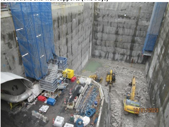
Figure 2 3 Ongoing excavation of the station box (Burwood North). Ongoing tunnelling in the adit.
