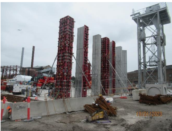
Figure 2 1 Ongoing large concrete pours for the Spoil shed foundations and wall supports (The Bays)
