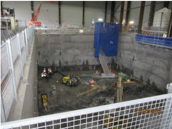
Figure 2-5 Ongoing excavation of the eastern shaft within the acoustic shed (Five Dock-east).
