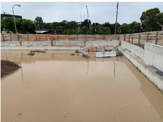
Figure 4.1: Westmead Site – Water accumulated on site to be transferred to onsite tanks, then to offsite water treatment
