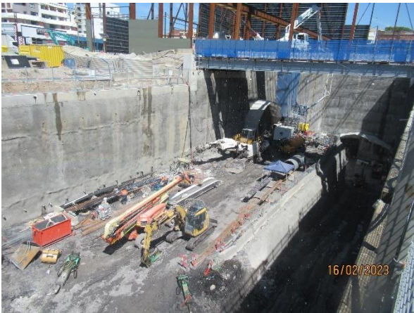
Figure 2-3 Commencement of tunnelling for the cross over cavern at the western end of the station box (Burwood North). Ongoing lining works in the adit.
