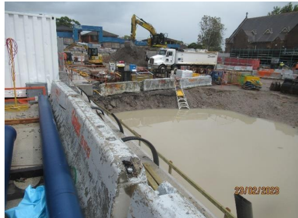
Figure 2-6 Commencement of excavation of the west shaft (FD). Load out of spoil.
