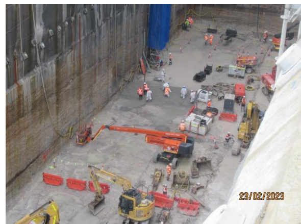
Figure 2 2 Concreting works at the base of the station box – western end (The Bays).
