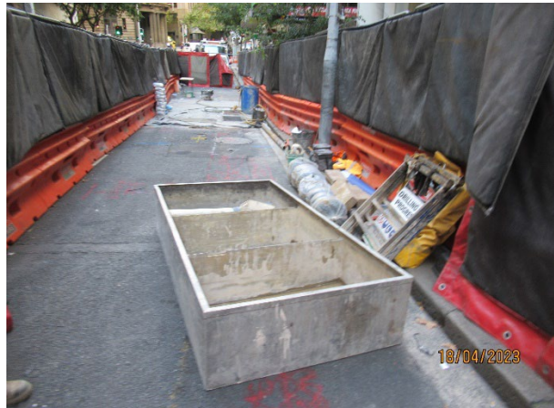
Figure 5 4 Hunter St West: Clean up after completion of geotechnical drilling activities in Hunter Street.
