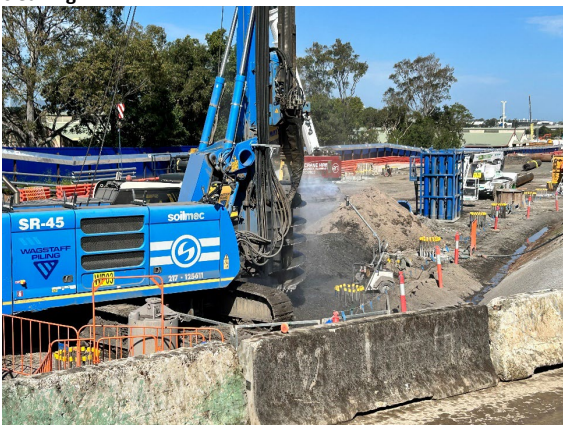
Figure 3.5: Clyde Dive site – Piling for the Dive Structure along the ATC boundary
