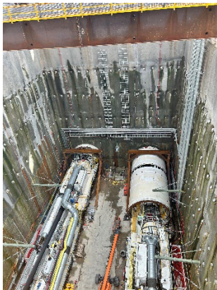
Figure 1 1 Tunnel Boring Machine on left commenced tunnelling during the reporting period. (The Bays)
