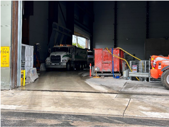
Figure 1.5 Ongoing excavation of the eastern shaft and loading of trucks within the acoustic shed (Five Dock-east).
