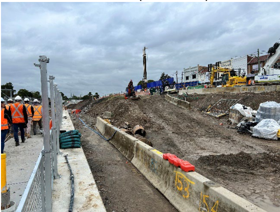
Figure 1.7 Piling on the top level of the station box at North Strathfield
