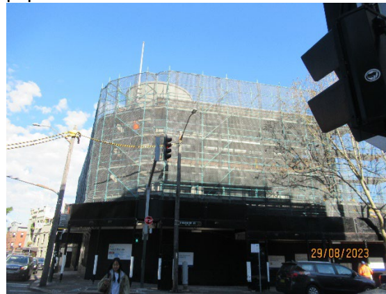
Figure 3.4 Pyrmont St West: Scaffolding installed around the building in preparation for demolition
