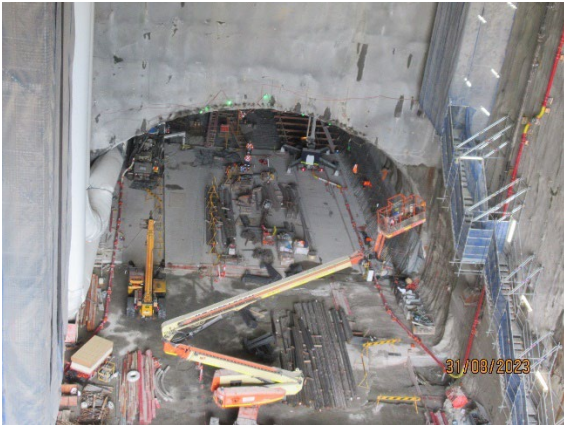
Figure 1.3 Concrete pour underway in the Cross Over Cavern at the western end of the station box (Burwood North).
