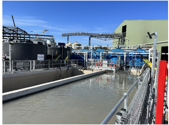
Figure 2.10: Rosehill Site – 50L/s Water Treatment Plant operating
