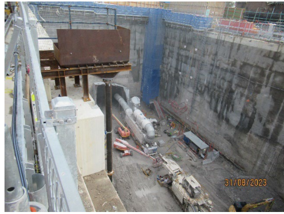
Figure 1.6 Commencement of excavation of the western cavern using road header (Five Dock-west).
