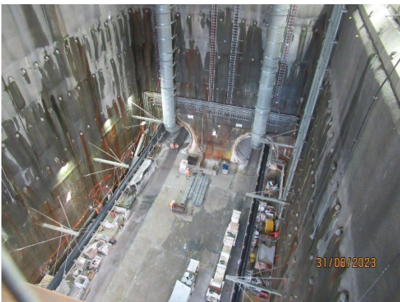
Figure 1 1 Base of the station box showing conveyors exiting tunnels (The Bays) and TBM support activities.
