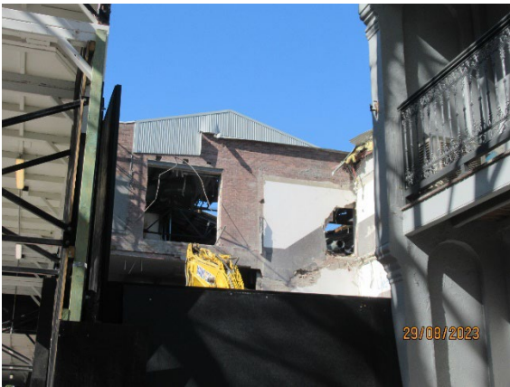
Figure 3.3 Pyrmont St West: Hard demolition of area near truck access from Pyrmont Street
