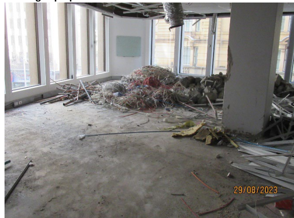
Figure 3.6 Hunter Street East: Ongoing soft strip; segregation and load out of wastes in the various buildings
