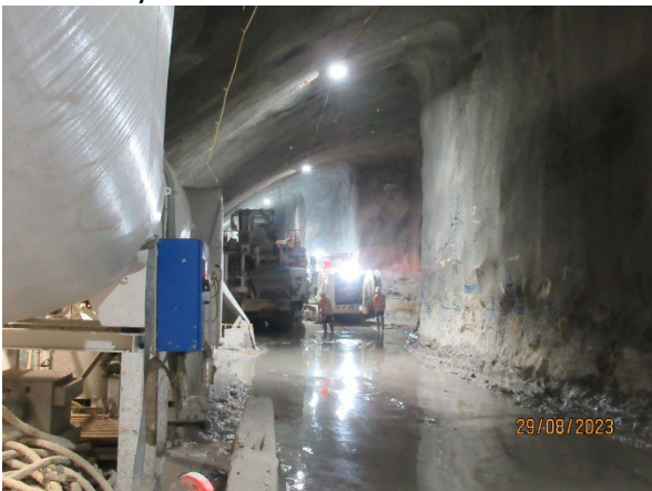
Figure 3.5 Station Cavern: Ongoing excavation of the southern heading by road headers and roof support
