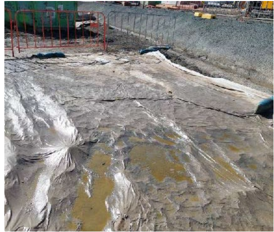
Figure 2.8: Clyde Dive site – Hydraulic oil spill in sediment controls
