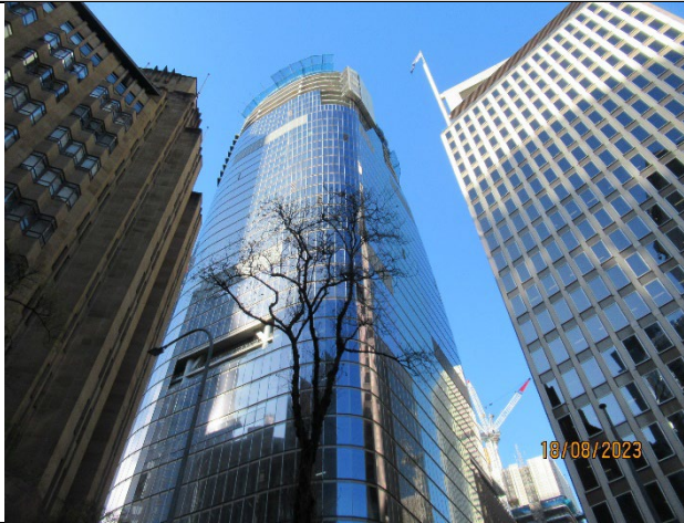
Martin Place North: View from corner of Hunter and Castlereagh Streets. Ongoing façade construction.
