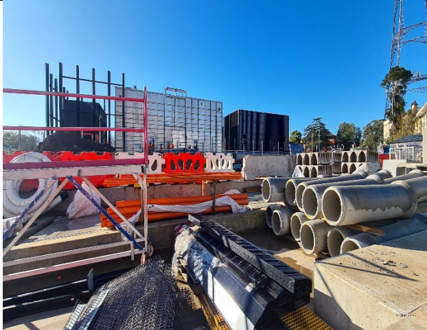
CDS: Installation of pipework and connections in progress for hydrant water tank.
