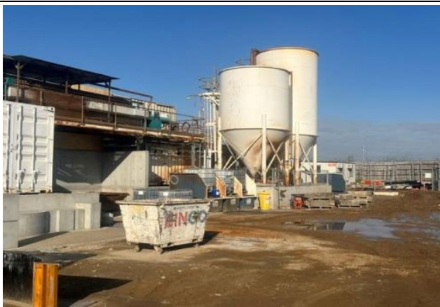
Ongoing operation of the WTP
