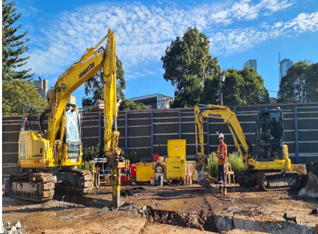
CDS: Trenching (hammering) works for stormwater connection underway. Observed operator wetting down work area during hammering (good practice)
