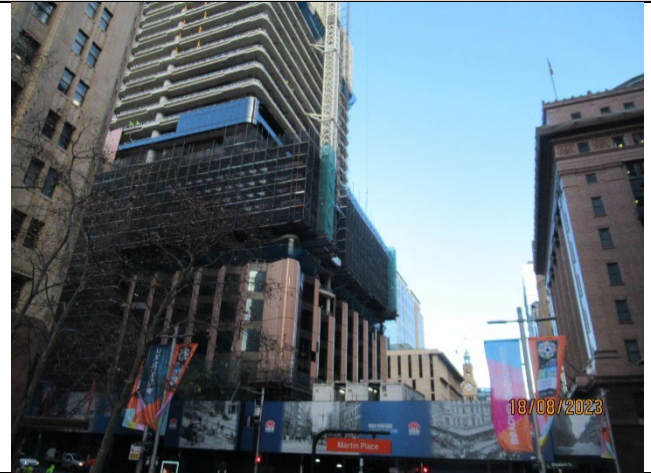
Martin Place South: View from Martin Place west of Castlereagh Street. Concrete pumping from Castlereagh Street.
