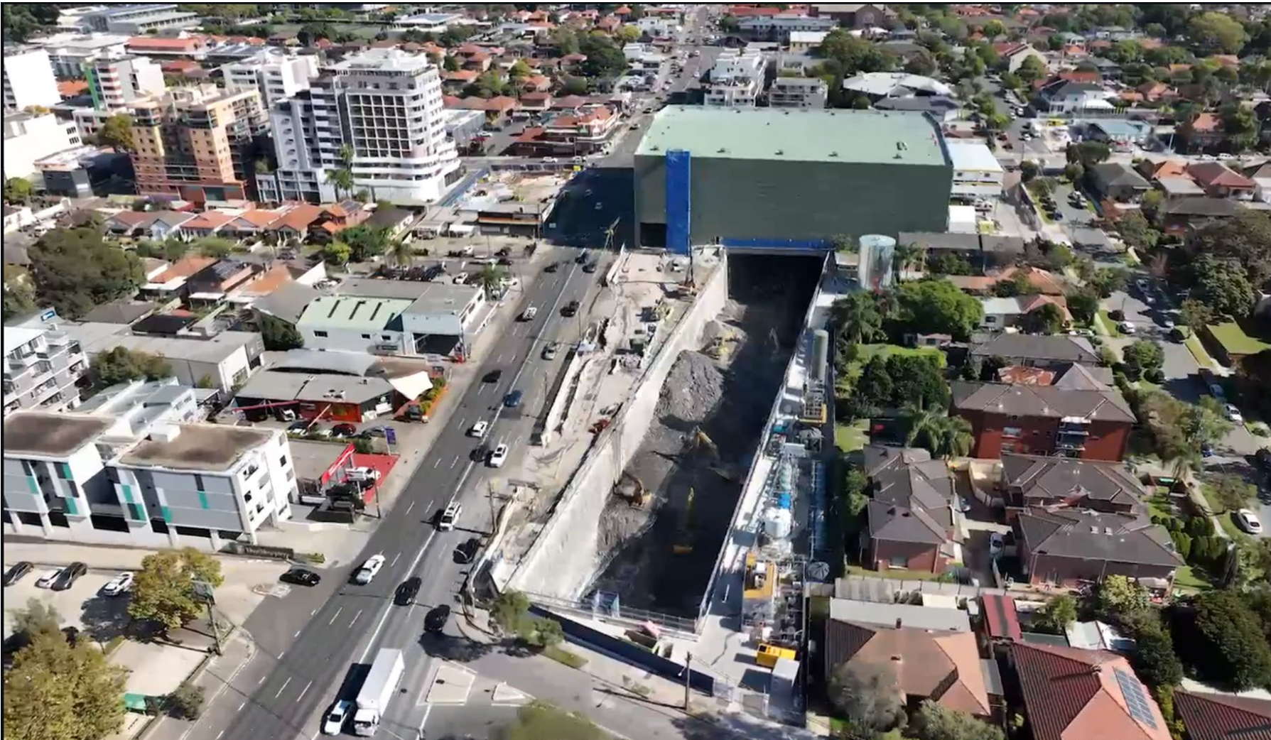
Figure 5-3 Burwood Acoustic shed and open station box excavation (looking west along Parramatta Road)
