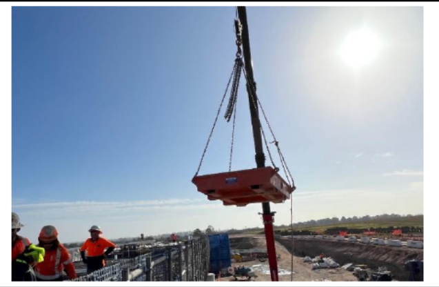
M12 Bridge - Trays are lifted onto the deck of the bridge for clean-up. At the time of the inspection housekeeping was noted to be very good
