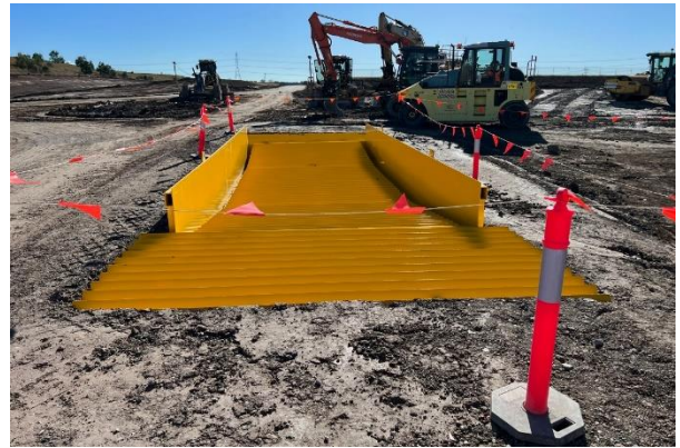
Patons Lane - A wheel wash has been installed however is not being used by the project. ER questioned why this was the case and asked CPBUI to implement additional controls
