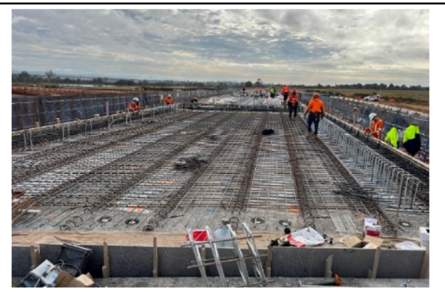
M12 Bridge - Deck pours are the remaining works on the M12 bridge
