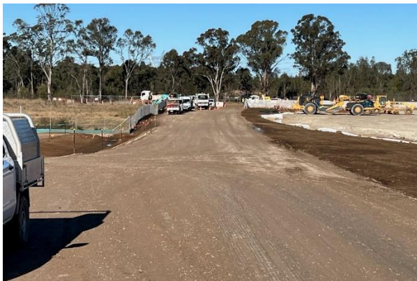
Patons Lane - The section of track from the wheel wash is meant to be sealed, however is not at this point in time. ER asked for a timeframe when this will be completed as this could be a key control in managing mud tracking
