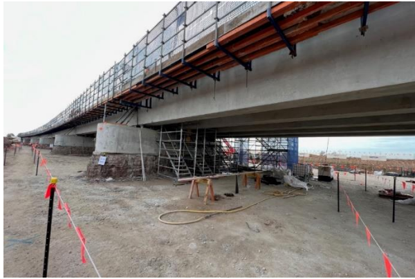
M12 Bridge - All super Ts have been installed on the M12 bridge, with deck pours remaining
