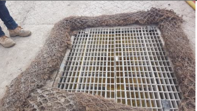
St Marys: Erosion and sediment controls at pit adjacent goods shed require maintenance.
