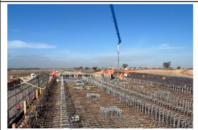
M12 Bridge - Concrete pours continue at the M12 bridge as it is finalised
