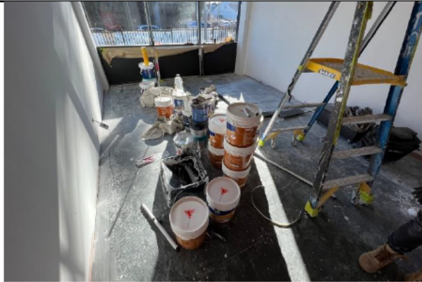
Painting has commenced on level 1, paint is generally being applied via rollers rather than spray. All paint is stored within the SPO
