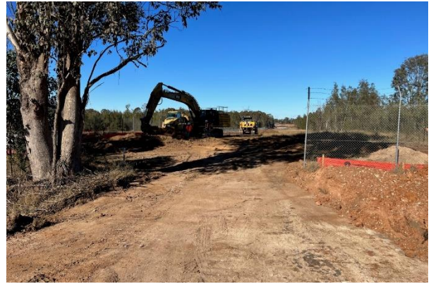
Defence Lane - The entry / exit point from the Defence site onto Patons Lane does not have appropriate wheel wash or mud tracking controls. Please install controls in this area
