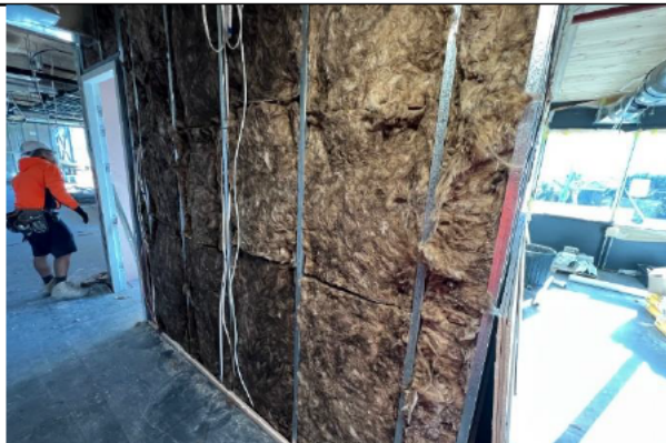
Earthwool is used as a sustainable acoustic treatment within the walls of meeting rooms
