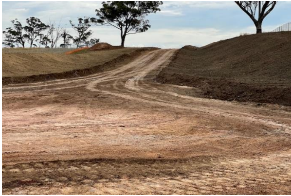
Luddenham Station - The disturbed areas at the Luddenham station round a bout have been stabilised with hydromulch, this is good practice
