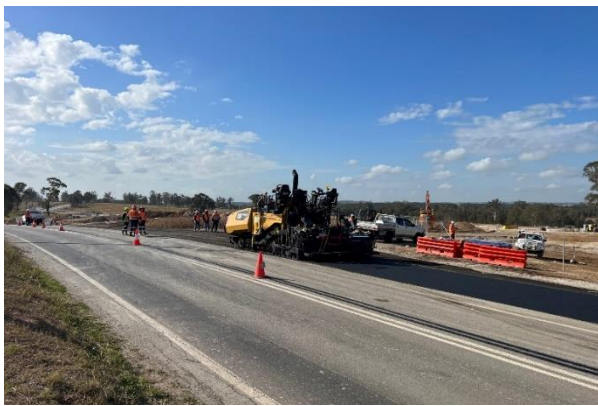
Luddenham South - Sealing works created a dedicated slip lane to and from the site
