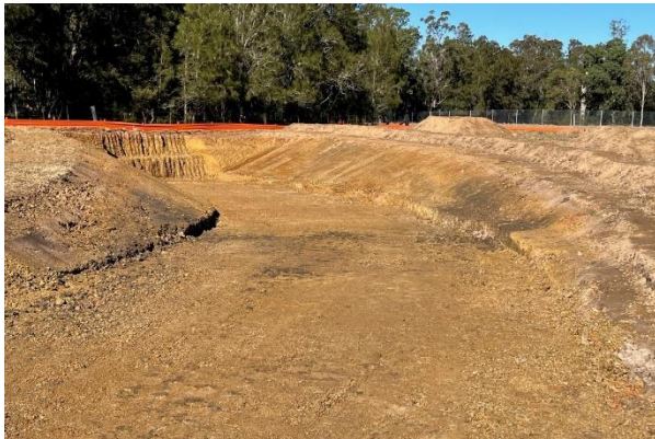
Luddenham South - The haul road has not broken through to Cosgrove's Creek yet and is acting as an additional sump
