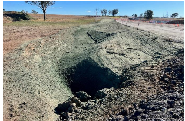
Luddenham South - The drains have been sprayed with hydromulch – this is good practice
