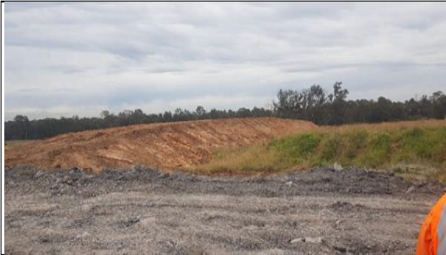
Bringelly Services Facility : Consolidated spoil, and ACM stockpiles well formed, awaiting seeding.
