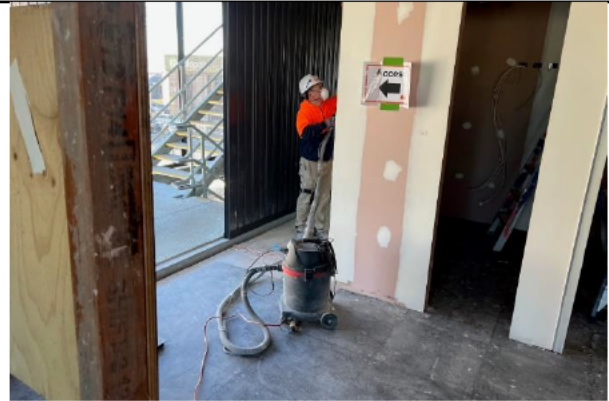
Dust from sanding is immediately vacuumed reducing the risk to the workforce and the environment
