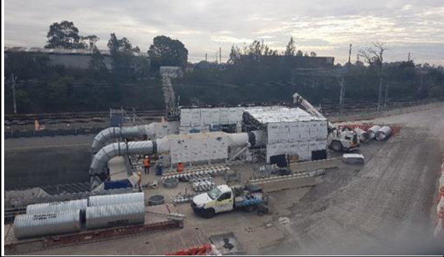
St Marys: Stub tunnel air extraction system noise mitigation (acoustic blankets) well implemented.
