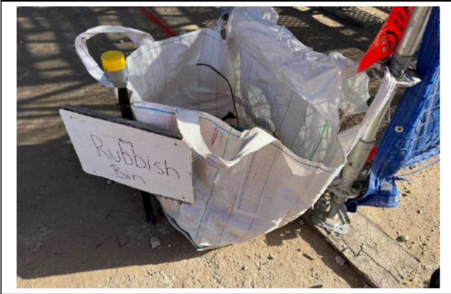
M12 Bridge - Waste bags are being reused as garbage bins, a simple but good reuse of materials
