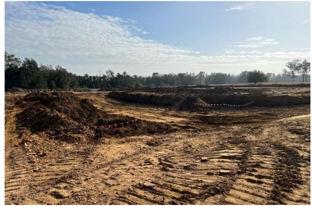
Cosgrove's Creek - Construction has commenced on the flood retention basin on the southern side of Cosgrove's Creek
