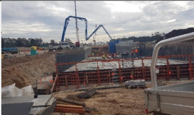
Orchard Hills: View north of dive structure base slab and FRP works, with box excavation beyond.
