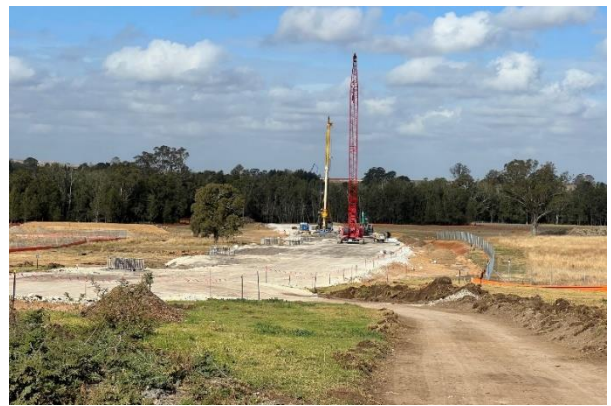
Luddenham South - Piling underway at Luddenham south making its way towards Cosgrove's Creek
