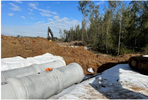
Defence Lane - The unnamed creek has been blocked off upstream while the creek crossing is being constructed
