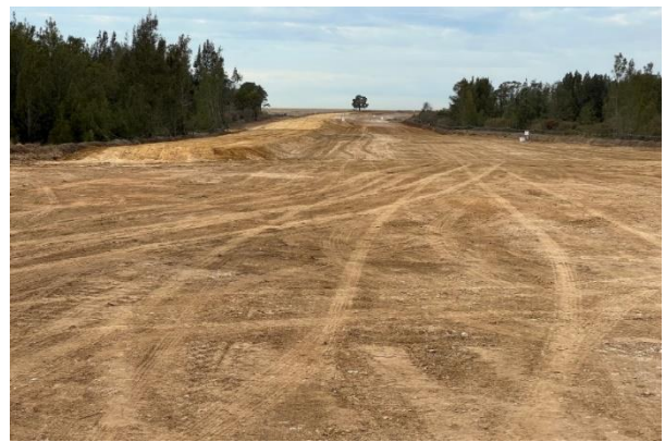
Cosgrove's Creek - The fine dust on the main alignment at Cosgrove's Creek needs to be monitored with dust suppression applied as required
