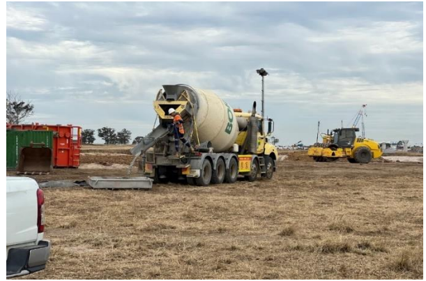
Luddenham Station - Concrete washout trays were in place and being used for the piling works
