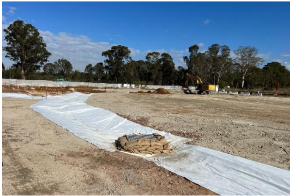
Patons Lane - Final ERSED controls have been constructed around the Patons Lane compound prior to handover to SSTOM
