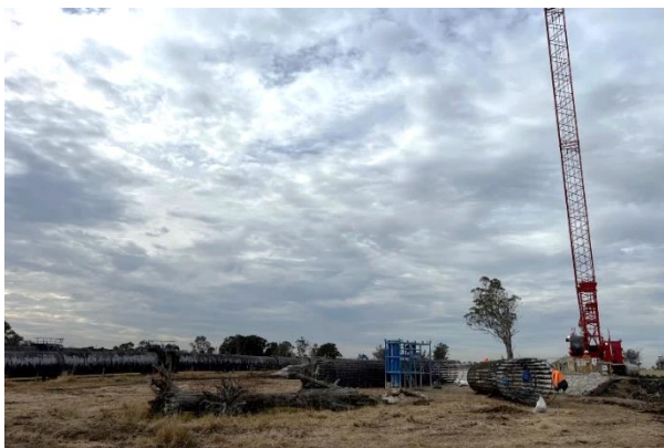
Luddenham Station - Piling has commenced within close proximity to the Warragamba pipelines
