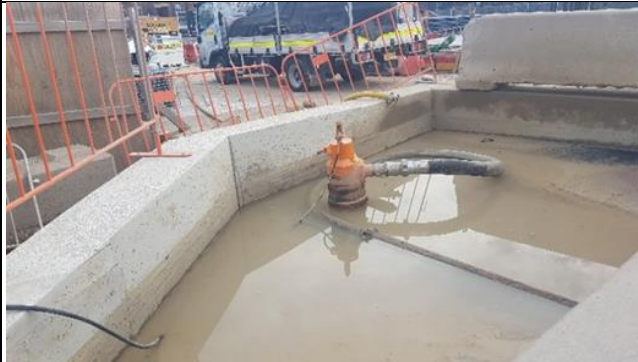
St Marys View north - South west Station St. sump and pump well managed, with CPBG to add CPESC recommended spill-over mitigation.
