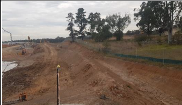
Aerotropolis view to southwest: Western clean water diversion swale to be completed.
