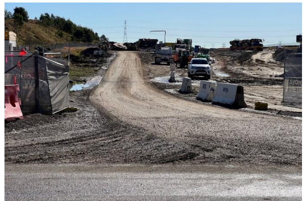
Patons Lane - There were no controls at the three entrance / exit points at Patons Lane to effectively clean mud from wheels. ER requested CPBUI to review all exit controls across the project and implement a proactive approach rather than a reactive one
