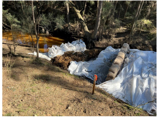
Cosgroves Creek - Cosgroves Creek has been blocked with a pump around to keep the works area dry and minimise the change of water pollution
