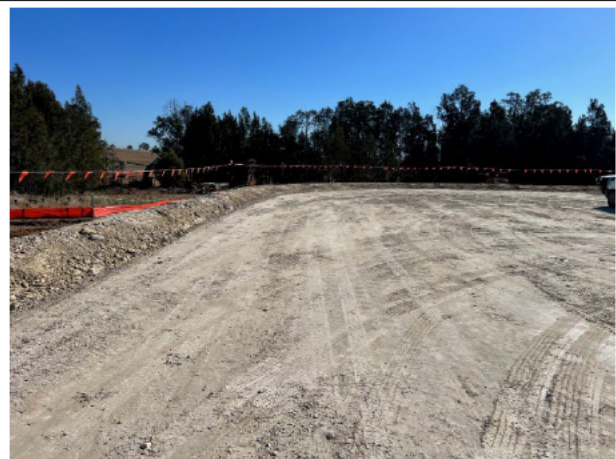
Cosgroves Creek A bund has been added to the top of the sandstone fill to prevent scour and runoff
