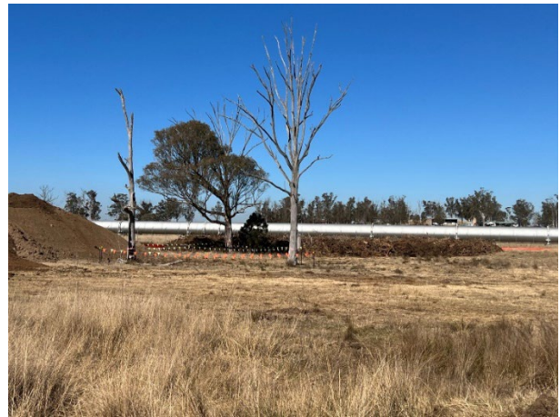
Defence - Mulch stockpiles have been nominated on the Defence land to be reused in the SSTOM works
