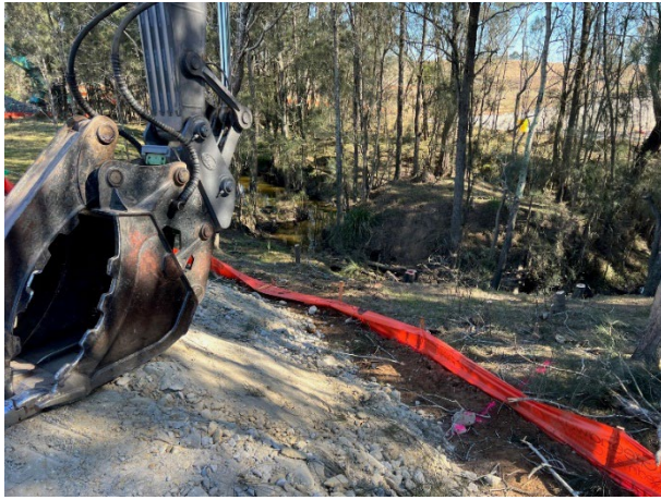
Cosgroves Creek - Tree removal across Cosgroves Creek is occurring to facilitate the viaduct structures
