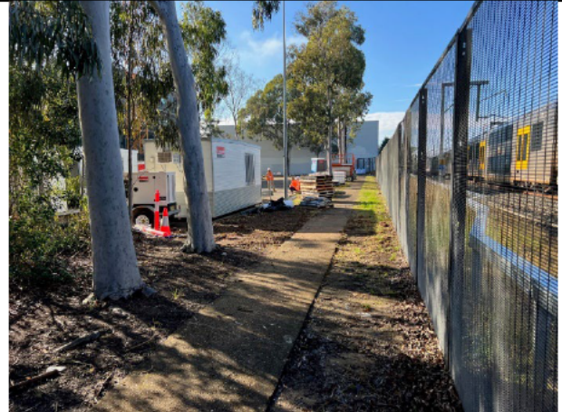
Initial sheds and equipment were brought onto the site compound area. Boundary screening and signage was not fully installed.
