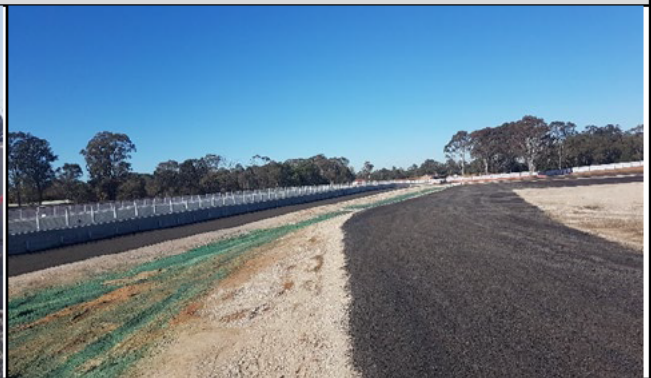
Lansdowne Rd. view south east – stabilization to be completed with a durable method.
