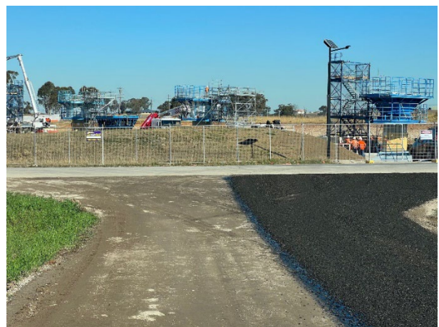
Luddenham North - The main entry / exit track at Luddenham North is in the process of being sealed
