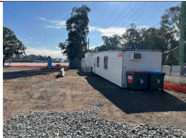
Site sheds have been setup at the Gipps St compound. Site screening and signage has been installed.
