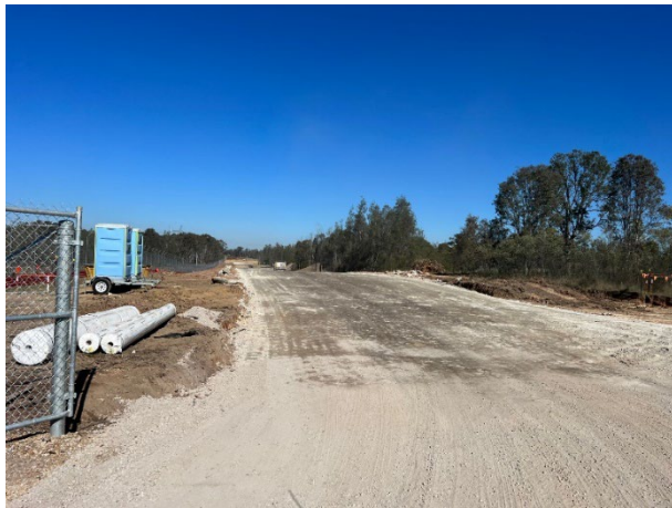
Defence - The entry to the Defence land has sandstone applied to it to minimise dust and a wheel wash has since been delivered for installation
