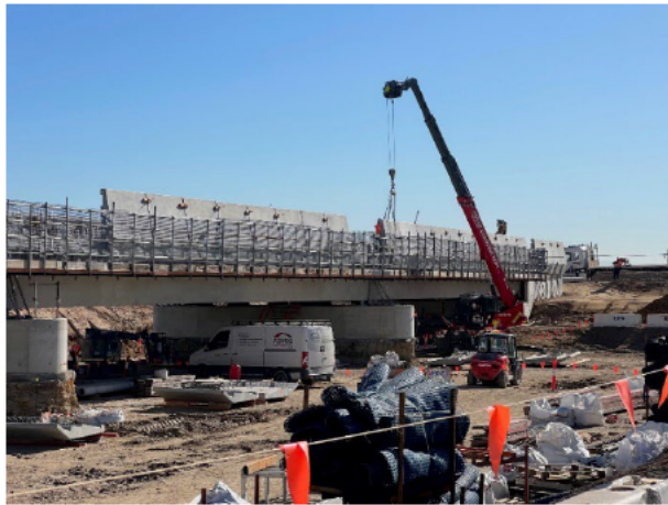
M12 Bridge- Parapets are being installed on the bridge structure before being handed over to the M12 contractor
