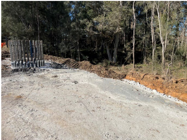
Luddenham South - Grout overflow from the concrete works on this pile has been stopped by the ERSED controls and was cleaned up
