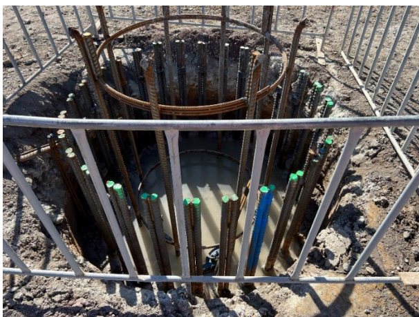
Luddenham North – Water from piling is captured and transferred to a treatment tank
