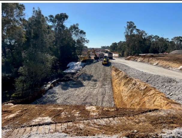
Blaxland's Creek'- Work continues on the creek crossing and the piling pad at Blaxland's Creek
