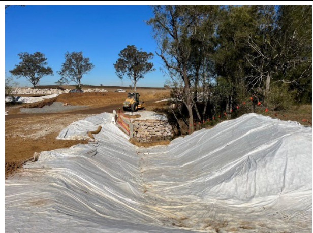
Blaxland's Creek - ERSED controls have been installed and maintained at Blaxland's Creek
