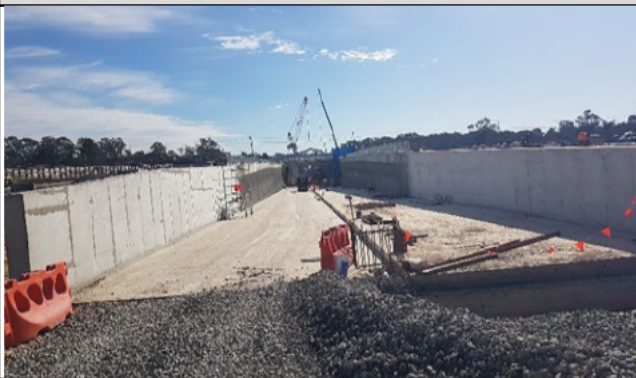
Orchard Hills: View north of completed dive structure and excavation under Lansdowne Rd.
