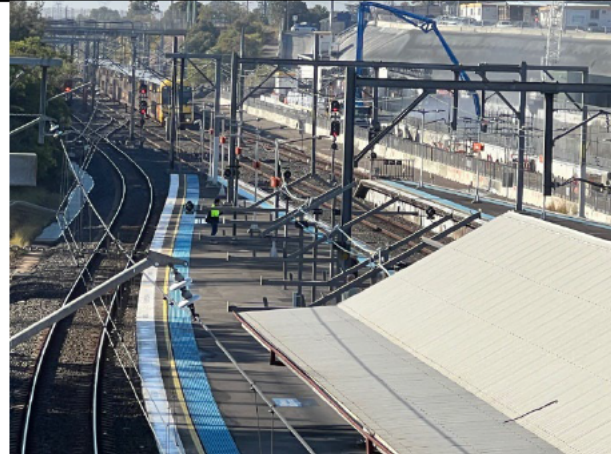
General layout of the works to sections of roofing have been removed
