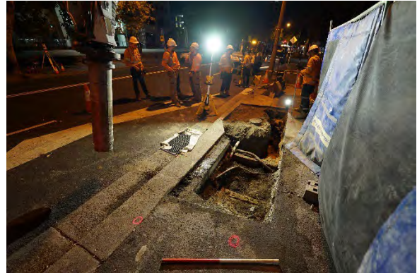
Figure 9 View northeast showing the exposed section of Town Drain with c20th century associated fills.
