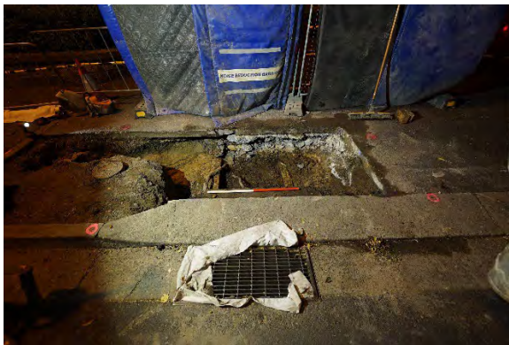
Figure 6 View north showing the Town Drain in relation to the modern stormwater grate.
