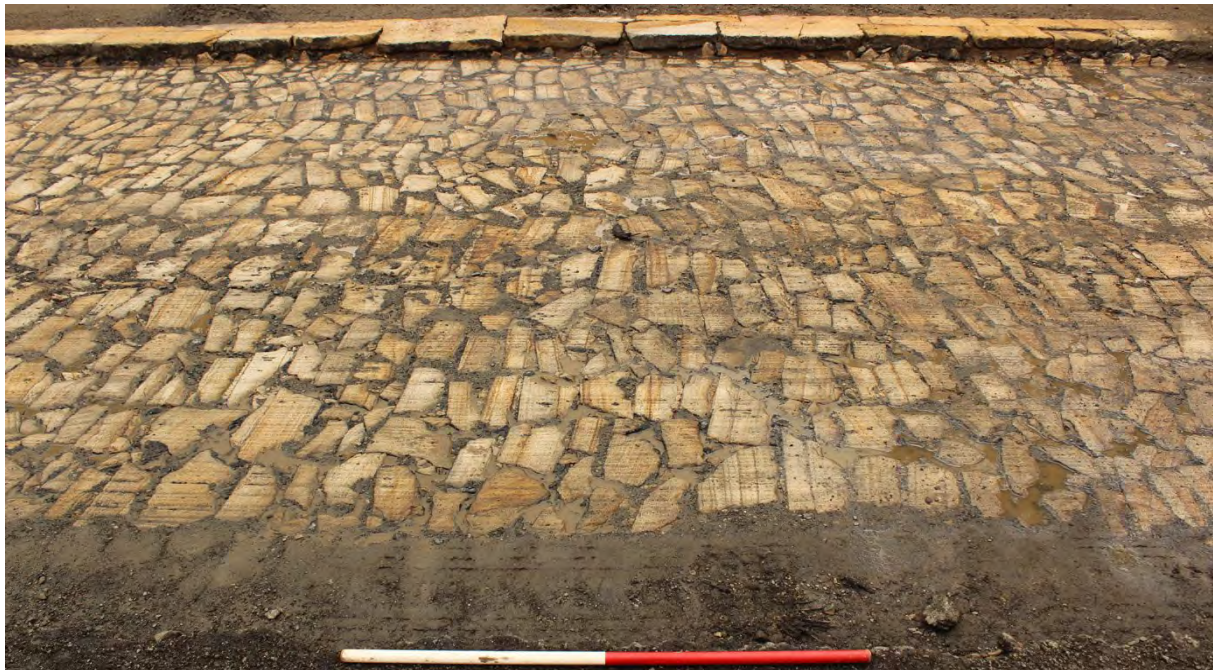
Figure 3.8 Example of truncated Telford Road surface showing the stone pavers or setts on Church Street. Scale is 1 metre.
