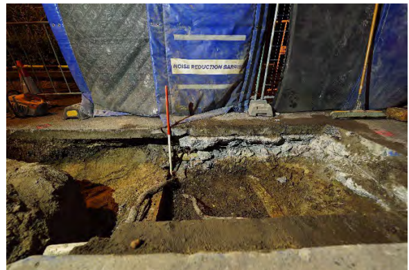
Figure 7 View south showing the depth of the Town Drain beneath the modern surface.
