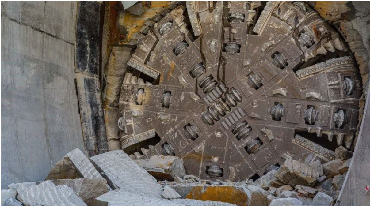
Figure 4-1 Photo of a tunnel boring machine at Epping Station on the Metro North West Line
