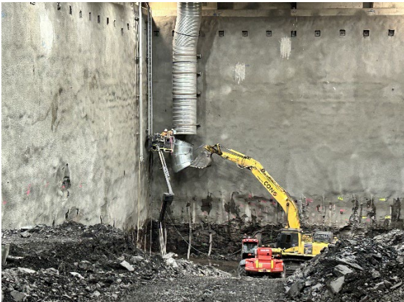
Figure 2.3: Westmead Site – Evening works being completed at eastern end of Station Box
