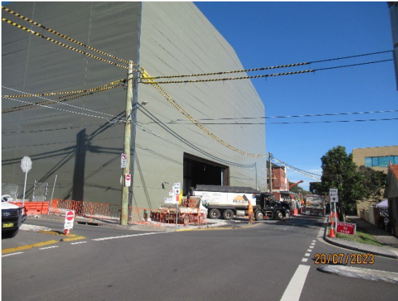
Figure 1.5 Improved use of the rapid shut door. (Five Dock-east). Vents now out of roof of the shed.
