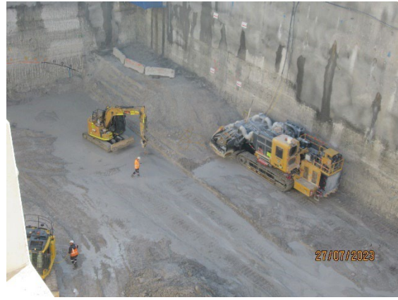
Figure 1.6 Ongoing excavation of the west shaft (Five Dock-west) utilising a surface miner as well as excavators with hammers.
