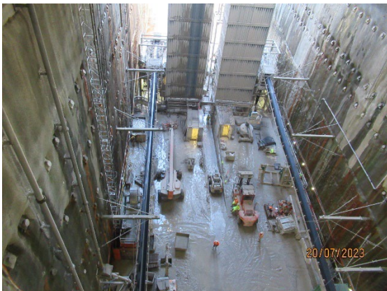
Figure 1 1 Base of the station box showing vertical conveyors in the background (The Bays). TBM support activities.
