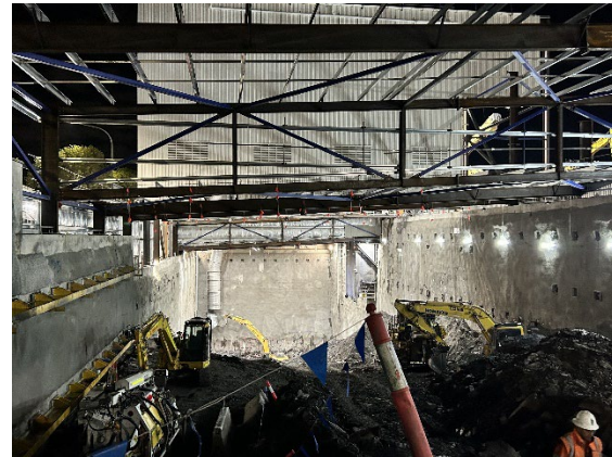
Figure 2.4: Westmead site – Evening works being completed at eastern end of Station Box
