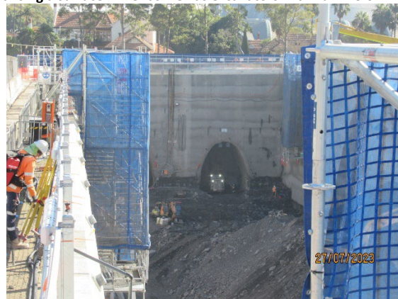
Figure 1.8 Excavation of the Station Box (SOP). Construction of nozzles in the western end.
