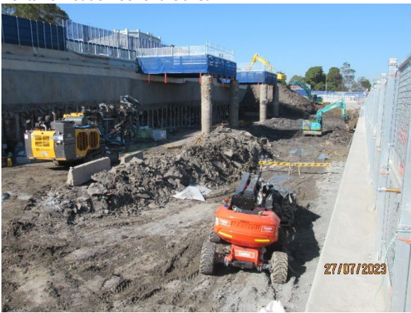
Figure 1.7 Excavation of spoil and wall support. Construction of load out platforms completed. (North Strathfield)
