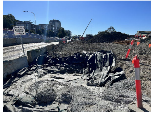
Figure 2.8: Clyde Dive site – Concrete Wash out requiring improvement
