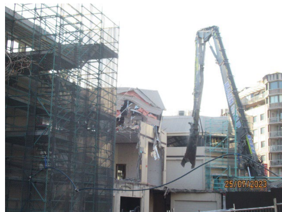
Figure 3.2 Pyrmont East: Ongoing hard demolition works using pulverisers or shears on long reach excavator
