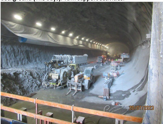
Figure 1 3 Excavation of the cavern at the western end of the station box under the acoustic shed complete (Burwood North).
