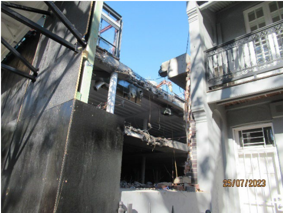
Figure 3.3 Pyrmont St West: Hard demolition of area for truck access using small Brokk excavator
