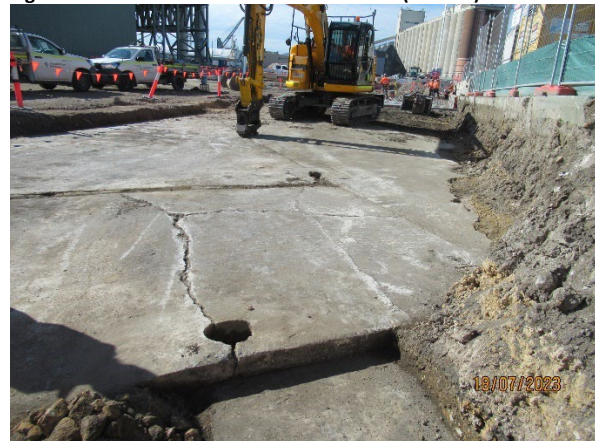
Figure 3.8 The Bays: Exposed slab from WWII era in footprint of the spoil shed
