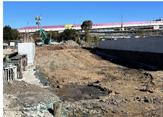
Figure 2.11: Clyde MSF Site – Mud tracking on Kay Street requiring improvement action
