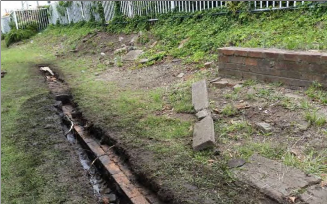
Plate 5: Platform at Hamilton Station classified as a ‘work’ by the project archaeologist, Wickham Transport Interchange project, 2015
