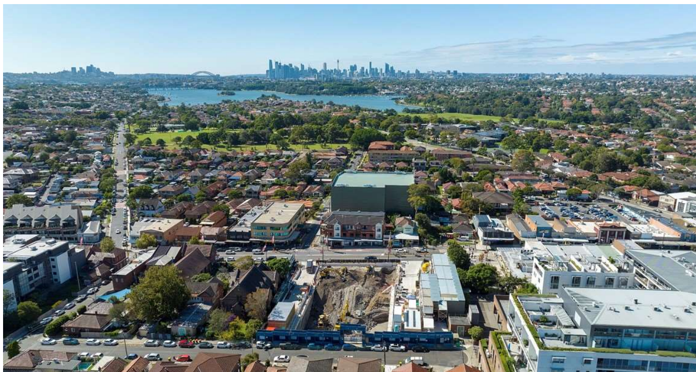
Figure 5-3 Five Dock east acoustic shed and Five Dock west site showing hoarding and site buildings.
