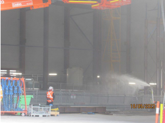
Figure 1 5 Water spray (mister) in use at the eastern shaft within the acoustic shed (Five Dock-east).
