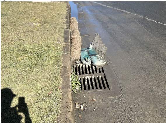
Figure 3.9: Clyde MSF Site – Stormwater Pit maintenance required on Unwin Street
