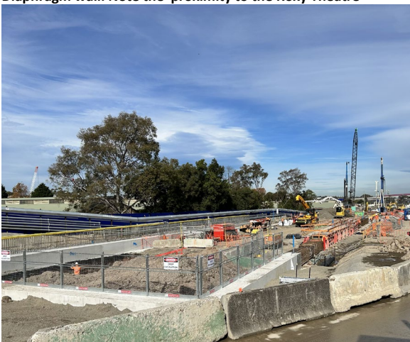
Figure 3.5: Clyde Dive site – Piling for the Dive Structure along the ATC boundary and Dive excavation commenced
