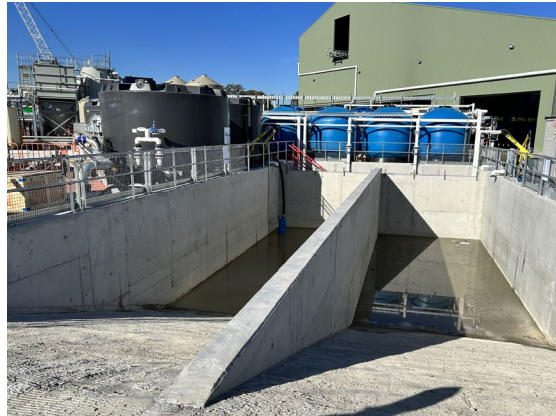
Figure 3.8: Rosehill Site – Long term Water treatment plant commissioning
