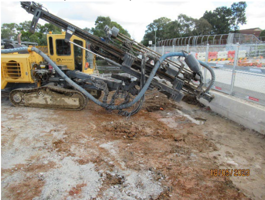
Figure 1.7 Rock anchor drilling for the capping beam at the western end of the Station Box (North Strathfield)
