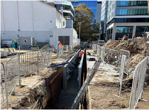
Figure 3.3: Parramatta Site – Guide wall construction for the Diaphragm wall. Note the proximity to the Roxy Theatre
