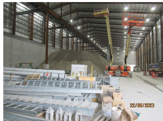
Figure 1 2 Ongoing cladding of the frame of the spoil shed. (The Bays). Use of the shed for storing spoil from the TBM.
