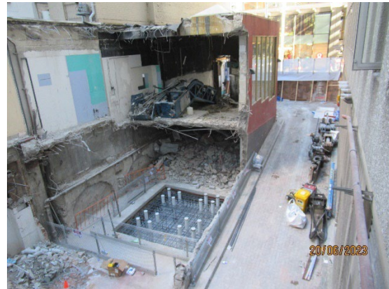
Figure 3.6 Hunter Street West: Tower Crane footing – hard demolition to allow for access to the footing.
