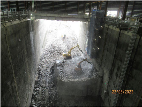
Figure 1.3 Excavation of the western end of the station box under the acoustic shed (Burwood North).
