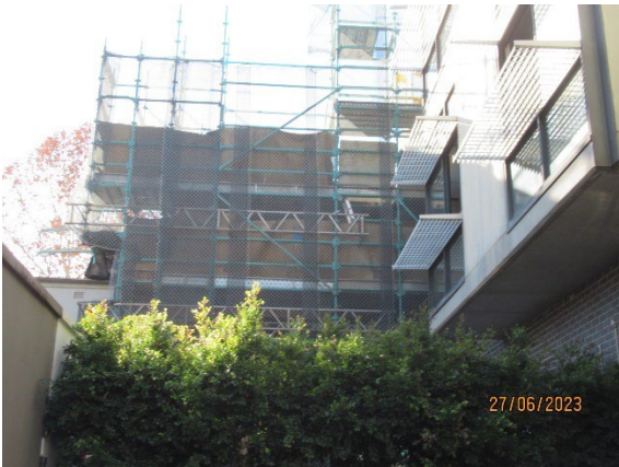
Figure 3.3 Hunter St West: Installation of scaffolding for area to be demolished for truck access.
