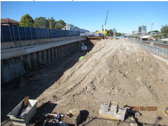
Figure 1.7 Excavation of some spoil and wall support. Construction of load out platforms. (North Strathfield)
