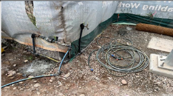
St Mays lift relocation - A small amount of grout was washed out in the corner of the site.
