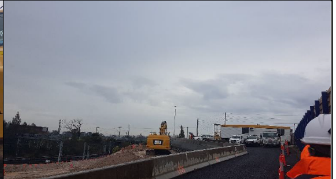
St Marys view east— Construction Accommodation and parking north of Chesham Road.
