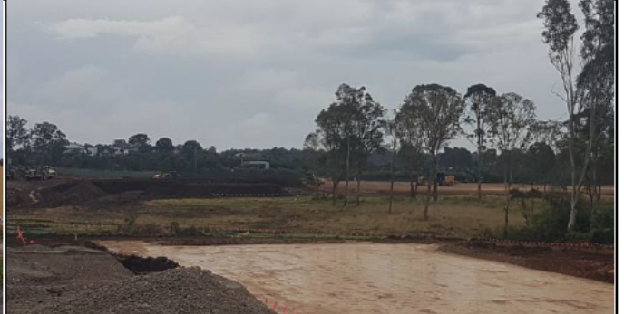
Orchard Hills view North - Preparation laydown areas (left) and precast tunnel segment storage pad (right)
