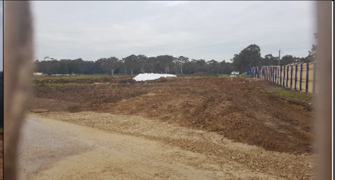
Orchard hills view south at diversion – Clearing south of Lansdowne Rd completed and hoarding on the right
