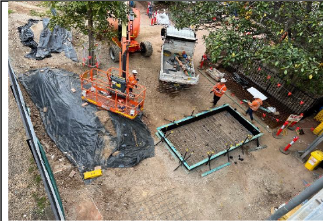
St Marys lift relocation – View of site to the south east from the concourse/ pedestrian bridge
