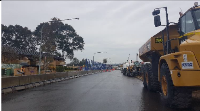
St Marys Station Road view west—Jersey barriers in place and Station St hoarding structure ready for panels.
