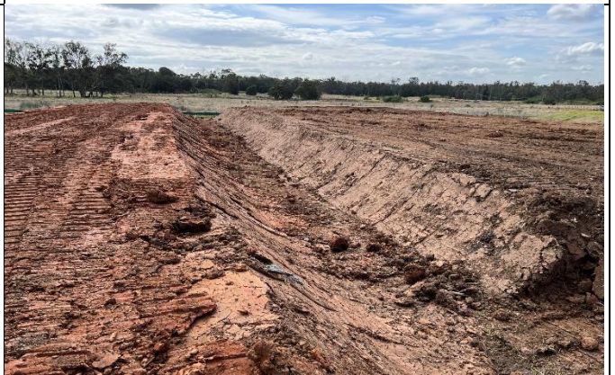
Bringelly Services Facility – View north from soil stockpiles west of central dam.
