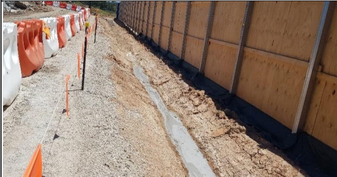
Bringelly Services Facility – Swale along Northern Boundary concrete fines discharged into swale
