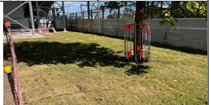
St Marys lift relocation - Landscaping commenced with planting of turf. The contractor to maintain this until project handover
