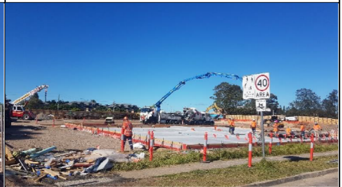
St Marys looking south west at Station plaza– Water Treatment Plant slab construction.
