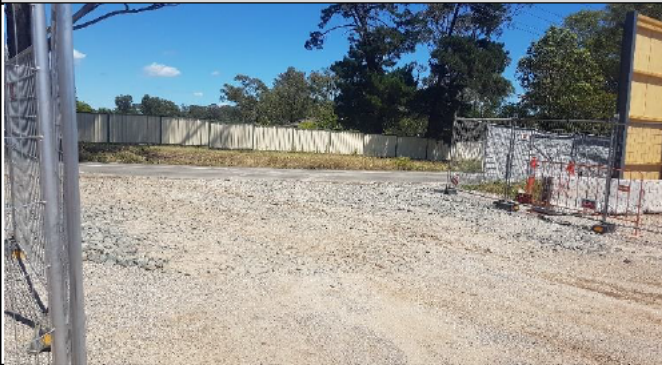
Orchard Hills north Kent Rd Access – Tracking indicated additional stabilised surface and rumble grid required
