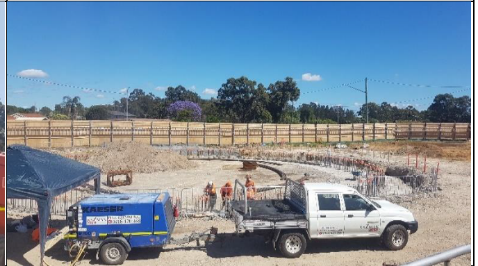
Claremont Meadows view west – shaft pilling and blinding complete with break-back underway
