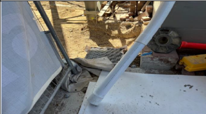
St Marys lift relocation – Stormwater from roof of the existing structures to be directed into live stormwater drainage lines
