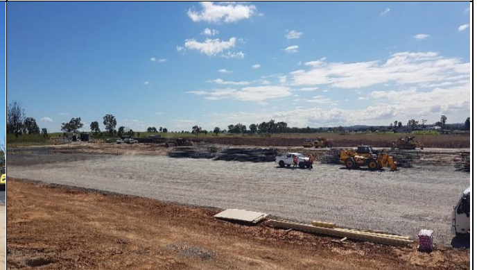
Aerotropolis : View south west from compound to low risk area pilling pad.
