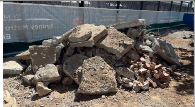
St Marys lift relocation – Concrete broken out was sent to concrete recyclers
