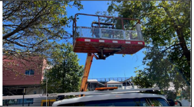
St Marys lift relocation – Care needed to be taken when parking equipment so it doesn't damage retained trees
