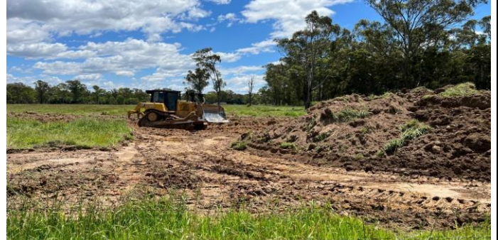
SMF - Works commenced on the large sediment basin on the northern end of the SMF
