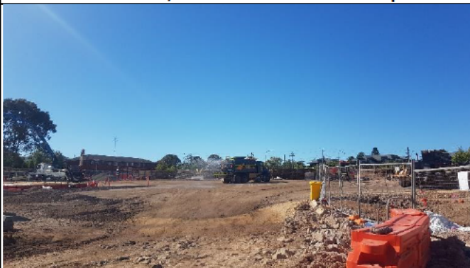
St Marys looking south east to Station Plaza – Water cart in action.
