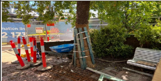
St Marys lift relocation – Tree protection has been installed and should remain until final works have been completed
