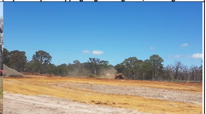
Orchard hills– view south at works South of Lansdowne Rd . Dust mitigation measures require improvements
