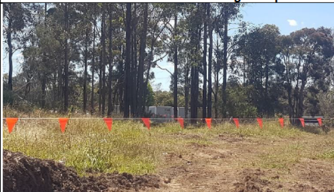
Orchard Hills – PCT segregation bunting requires appropriate signage
