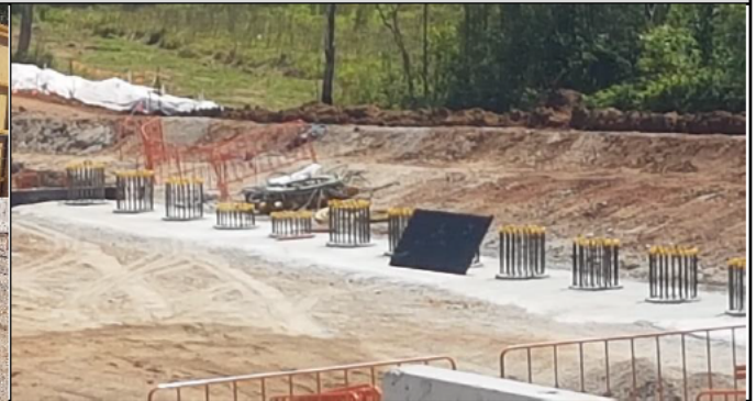
Orchard Hills north – Pile blinding and break- back. A hydraulic pile crossing ring is being used, reducing noise
