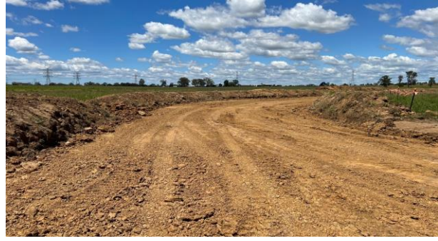
SMF - Windrows formed on the perimeter of haul road , acting as dirty and clean water diversions
