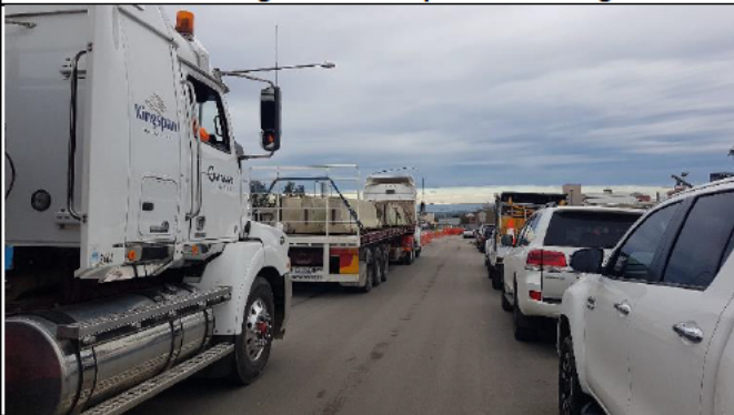
St Marys – Delivery and installation of jersey barriers in preparation of closure of Station St west bound lane.
