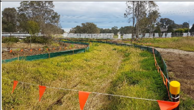
Orchard Hills view to Kent Rd - Erosion and sediment controls and bunting installed to protect drainage lines
