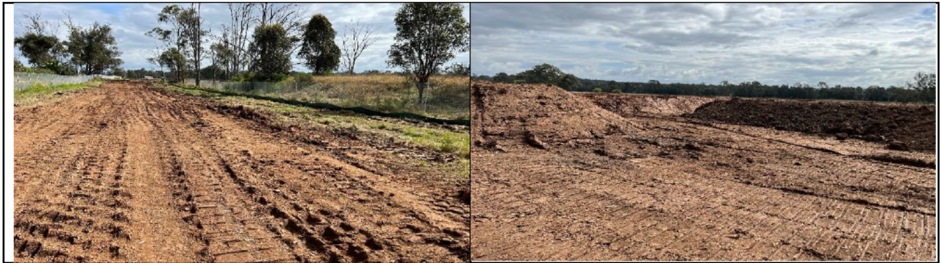
Bringelly Services Facility – View West of haul Rd between dam and southern boundary.
