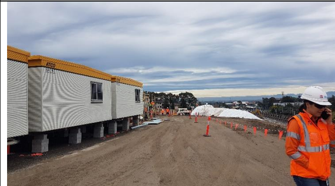
St Marys – Installation of accommodation and amenities at Glossop St entrance note unexpected find asbestos contaminated soil covered
