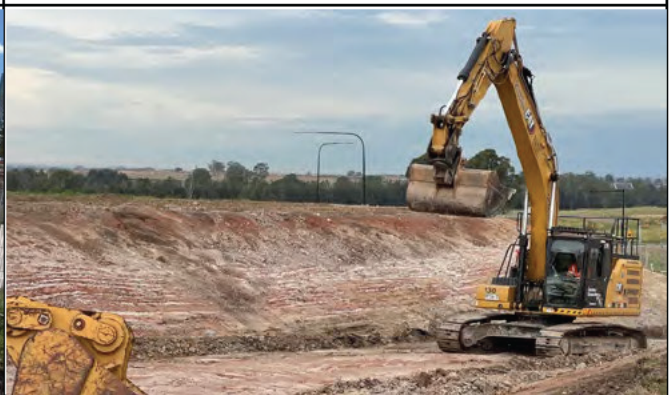
Luddenham Station – Works continue on the Luddenham station light vehicle access track
