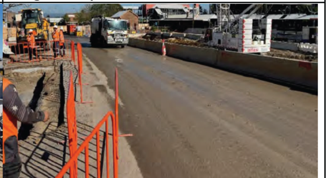
St Marys The internal sealed roads had significant mud deposition, however it is noted that a street sweeper was present to clean these roads
