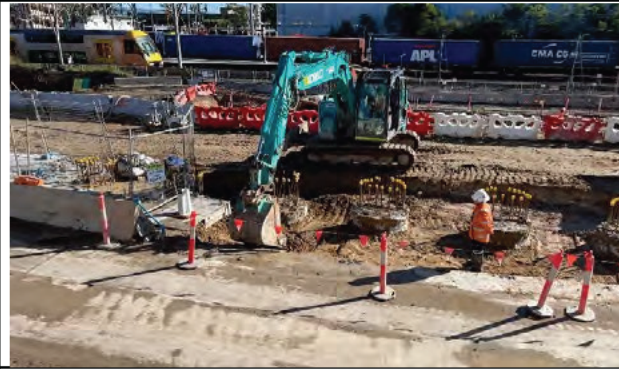
St Marys Piling and breakback continue at the central St Marys site
