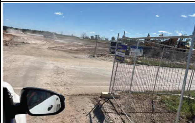
Luddenham Station - Dirt tracking was observed from the site to the private asphalted road.
