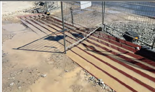
Orchard Hills south of Lansdowne Rd – The rumble grid is contributing to mud tracking
