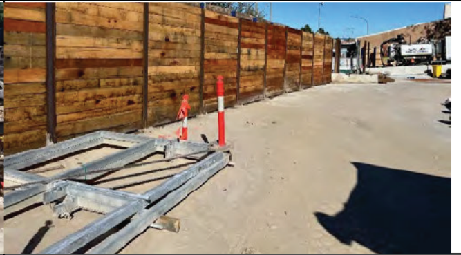
St Marys The hoarding has been completed at the station plaza area
