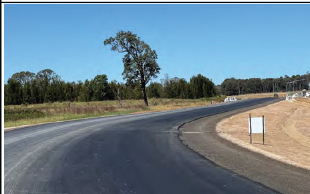
Elizabeth Drive – The access from the compound to Elizabeth Drive has been sealed which has resulted in no mud tracking on public roads.
