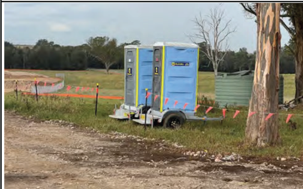
Luddenham Road South – Two portaloos have been placed within the tree protection zone
