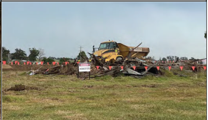
Luddenham Road South - Unexpected asbestos waste has been found on the site
