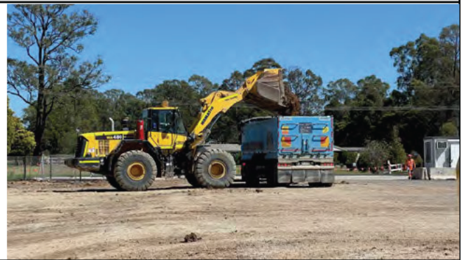
Orchard Hills north, view south – Spoil is being transported from Orchard Hills to the SCAW SMF
