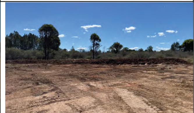
M12 to Consgroves Creek - Mulch has been formed into windrows on the perimeter of the site to separate clean and dirty water
