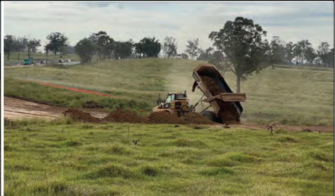
Luddenham Road South - Dust was observed during moxy operations at Luddenham Rd South
