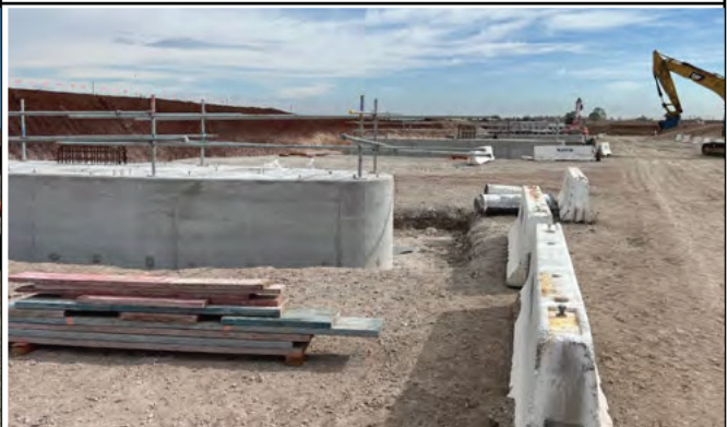
Elizabeth Drive – The pile caps at the poling pad are complete, ready for Super-T placement
