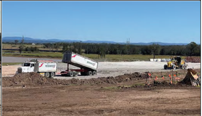
SMF - The internal haul roads and works areas are being filled with crushed sandstone to minimise dust
