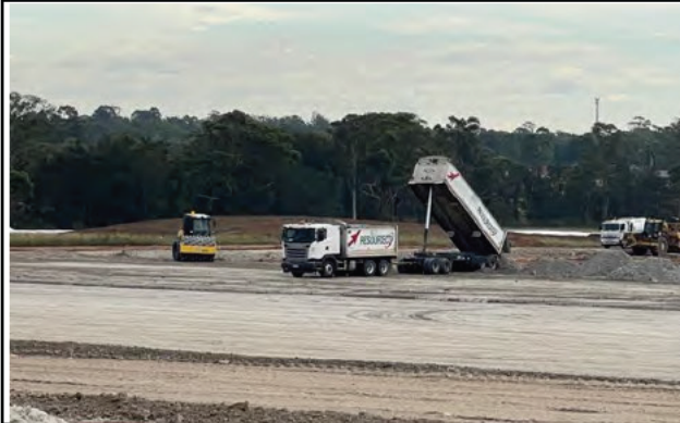
SMF - Sandstone deliveries continue to the SMF during approved normal construction hours
