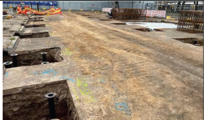
Dirt was deposited on the hardstand area. ER suggested programming this type of work with consideration of rainfall
