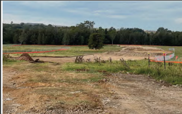
Luddenham Road South - ERSED controls have been placed around the Luddenham Road South alignment
