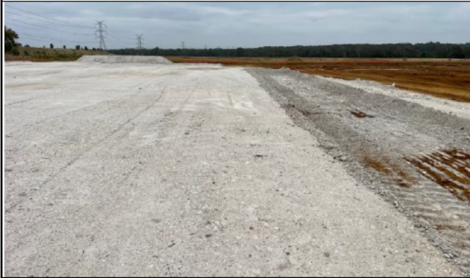
SMF – Crushed sandstone is starting to be spread out in the SMF
