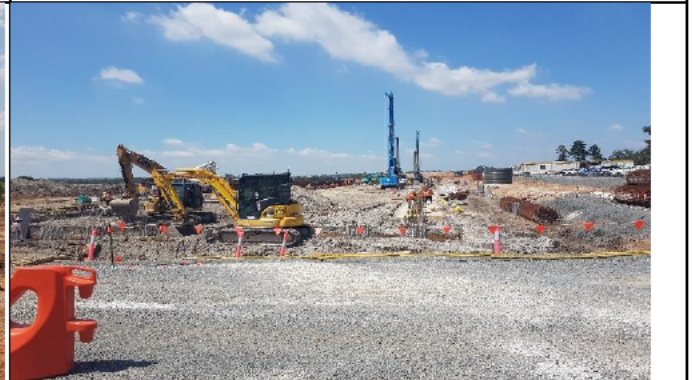
Aerotropolis : View north from entrance of DSI low risk area pile break back, blinding and capping beam FRP.
