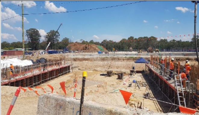
Orchard Hills view south – Capping beam FRP at Lansdowne Rd for bridge over station box.
