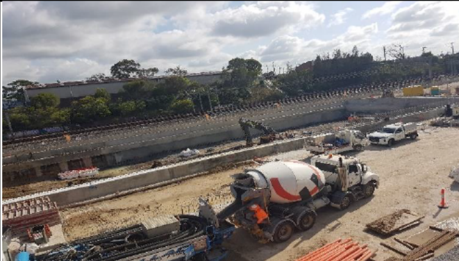
St Marys: View of works to the north showing eastern capping beam and station box excavation
