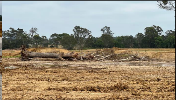
SMF - Trees have been cleared in the SMF with the remained needing ecologist supervision
