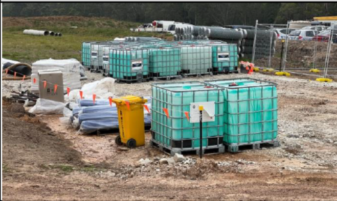
Patons Lane – Polymer compound has been ordered and used on site as an ERSED control
