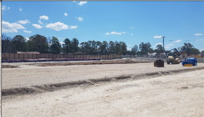
Orchard hills– view south at pilling pad preparation South of Lansdowne Rd .
