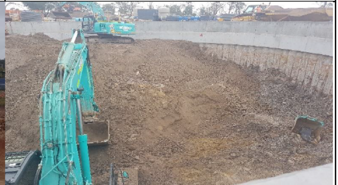
Bringelly Services Facility – Services shaft bulk excavation. Note completed capping beam and upstand
