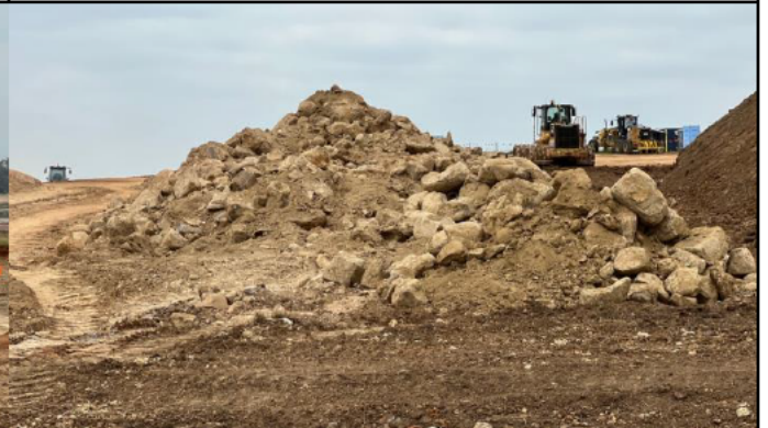
Elizabeth Drive – Rocks and boulders have been stockpiled for use in future ERSED controls
