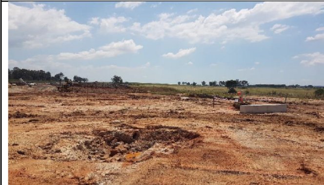
Aerotropolis : View southwest of surface soil stripping and asbestos removal in DSI moderate risk areas.
