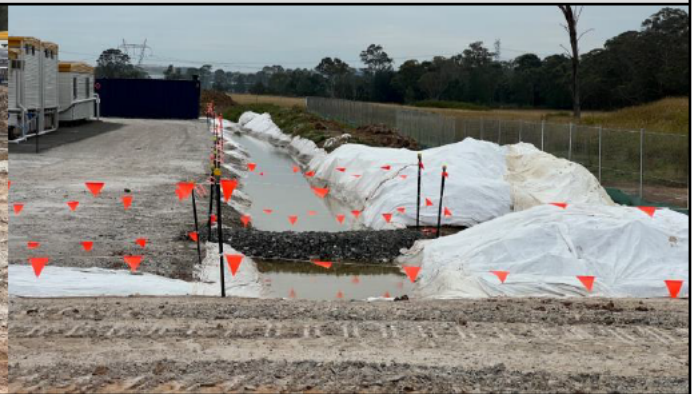
Patons Lane – The perimeter controls around the compound have been established and work as intended
