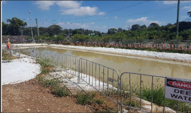
Claremont Meadows – View southwest along Great Western Highway of basin in operation
