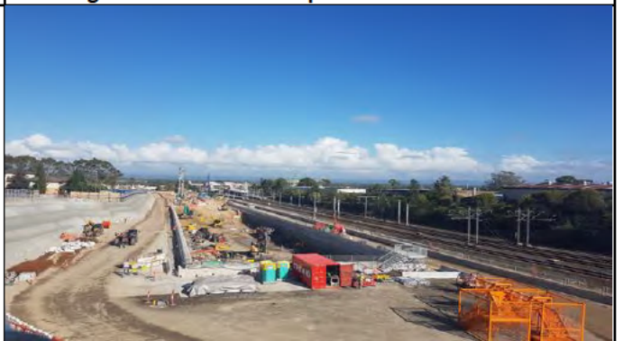
St Marys looking west - General view, with eastern station box in the foreground and piling at western extent.
