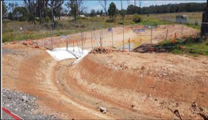
Bringelly Services Facility view north west–. Sed. Basin in operation and emptied
