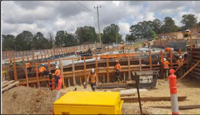
Orchard Hills view west – Bridge deck and abutting walls FRP ongoing at Lansdowne Rd bridge over station box.
