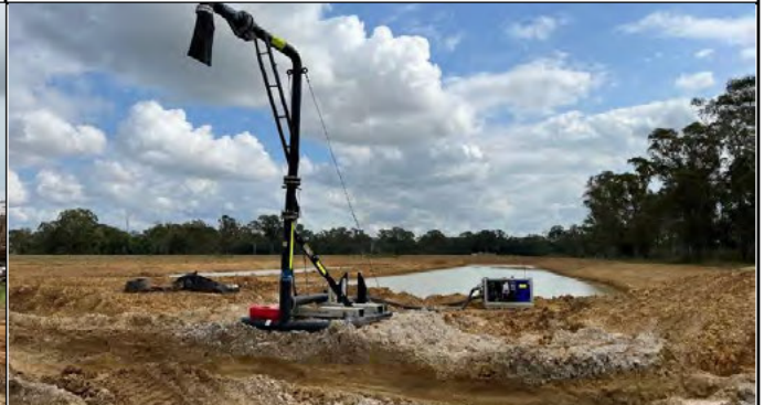
SMF - A pump and stand pipe has been set up at the 12ML basin to fill up the moxy watercarts
