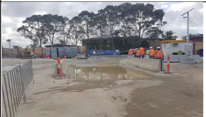
St Marys Main (Station Plaza) Laydown area : Eastern rumble grid / wheel wash in operation and effective.
