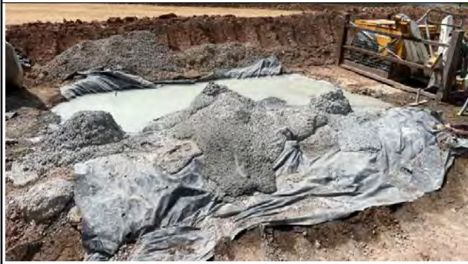
Elizabeth Drive – the concrete washout was inadequate and needed rectification.
