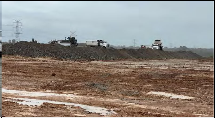
SMF - Sandstone material transferred from the site at Patons Lane to the SMF during construction hours
