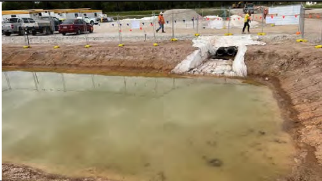
Patons Lane - The sediment basin at the compound is effective, with a lined outlet.
