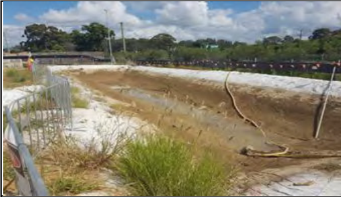
Claremont Meadows – View southwest along Great Western Highway of basin in operation and emptied
