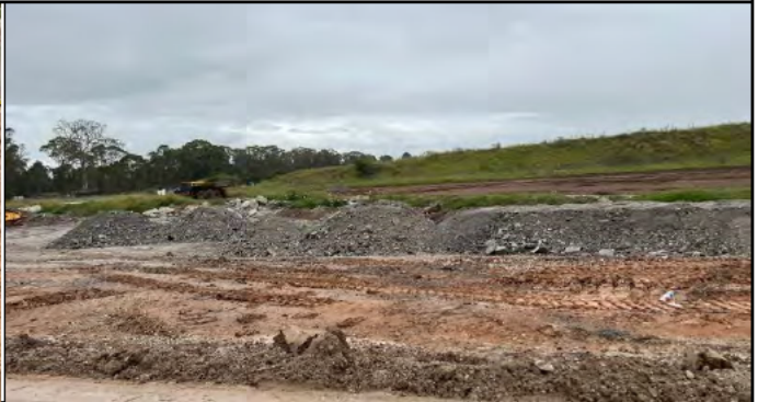
Patons Lane - Sandstone is being brought into Patons Lane out of hours
