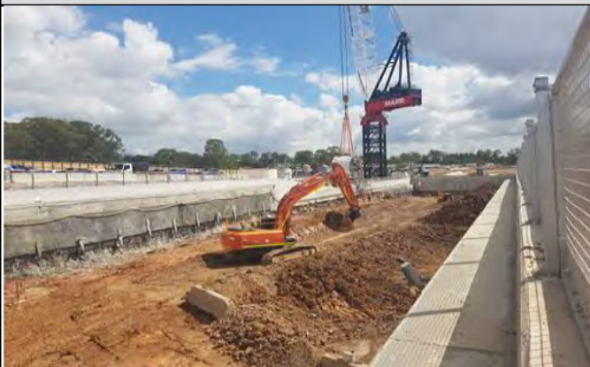
Orchard Hills Station box North – Station box excavation, shotcreting and soil nail installation within capping beam
