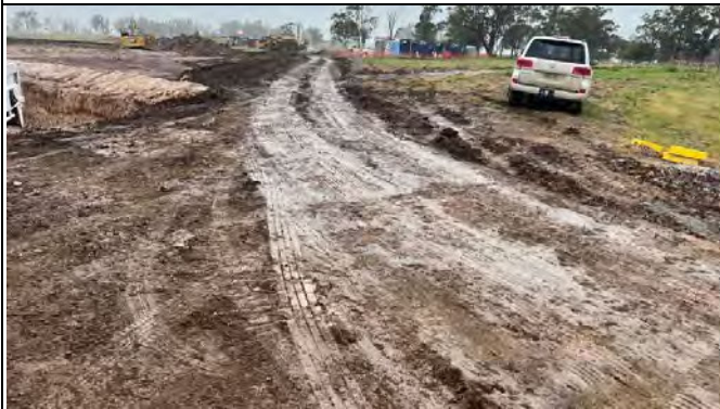
Luddenham Station – Earth access track needs to be stabilised all weather access track
