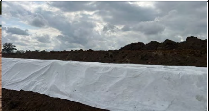
SMF - New windrows formed are stabilised with either compaction, polymer or geofabric
