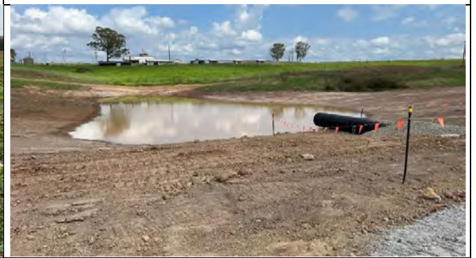
Elizabeth Drive - Pipes installed across the haul roads to allow flow from the M12 site to existing farm dams
