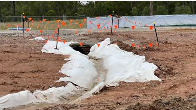
Patons Lane - Controls are being re routed to suit change in levels
