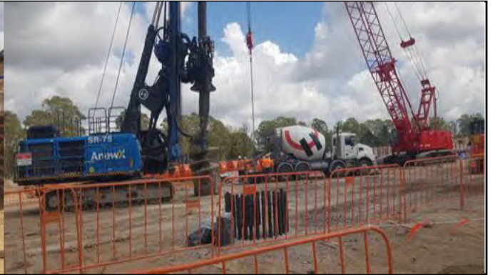
Orchard hills- view northwest of piling works in dive area south of Lansdowne Rd .
