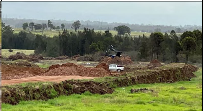
M12 to Cosgroves Creek - Recently cleared vegetation is being mulched or retained for future reuse
