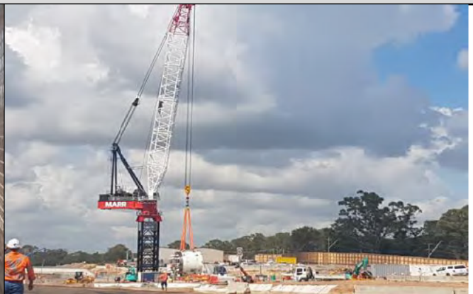
Orchard Hills north, view south – Tower crane used for TBM cutting head assembly, and storage on central western tunnel segment storage area.
