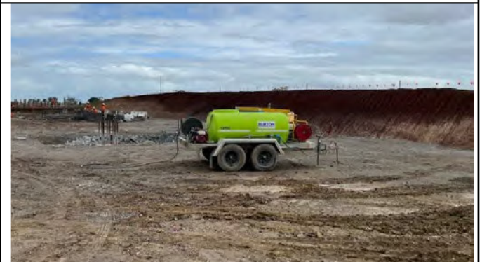
Elizabeth Drive - Water tank used to collect and reuse water within the site
