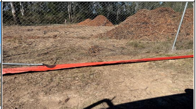
Patons Lane - Sections of sediment fence at defence land need re-instatement
