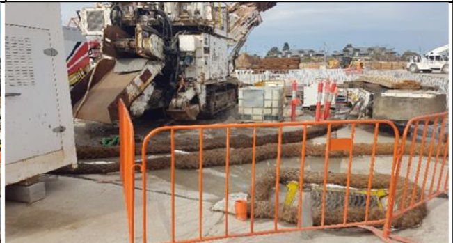
St Marys: Sediment accumulations noted and at sediment controls and in areas upgradient of live stormwater pit in the NW of the laydown area
