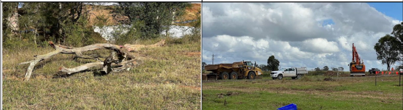
SMF – After completion of the temporary creek crossings felled trees with hollows to be relocated SMF - Retained trees at the northern end require segregation with fencing and signage.
