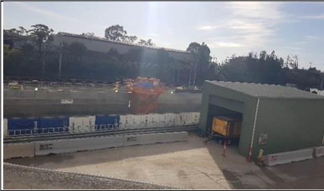
St Marys: Noise blankets well installed along southern and eastern capping beams and upright
