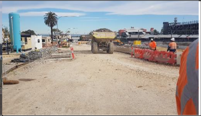
St Marys: Appreciable tracking noted on Station St onsite from spoil haulage on unstabilised road.
