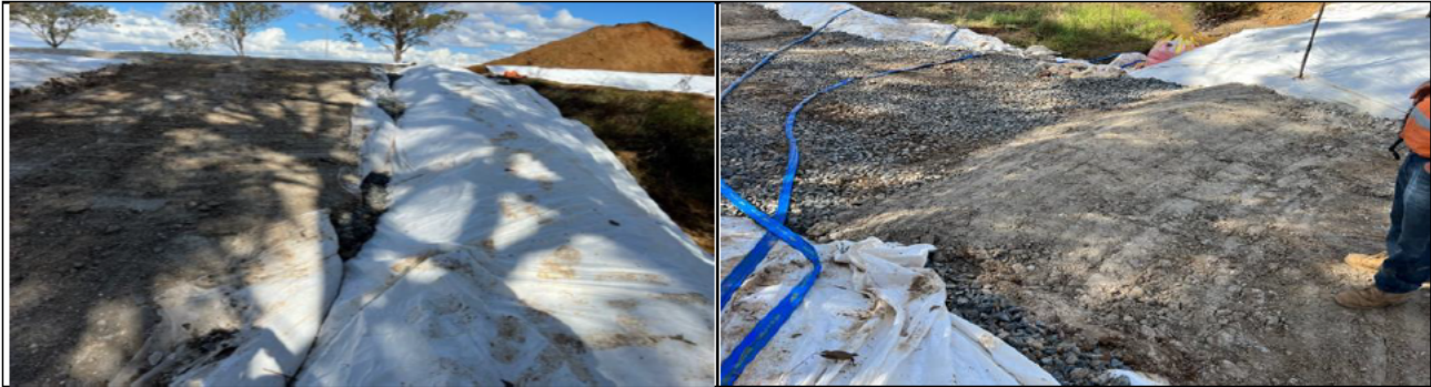
SMF - V-drain checks have been placed in the temporary crossings of Blaxland Creek SMF - Roll-over berms installed at the Blaxland Creek temporary crossing –good practice
