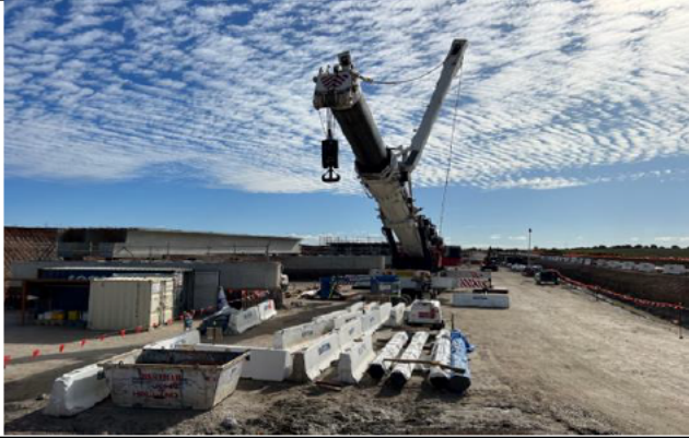
M12 Bridge - 650t crane has been mobilised to lift the remaining super-Ts into position
