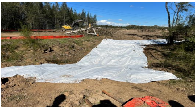
Patons Lane - Temporary creek crossing installed across the unnamed creek in the Defence Land
