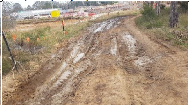
Orchard hills– Internal access north of SB3 from station box to SE laydown area needs stabilising
