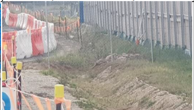
Bringelly Services Facility northern swale – Southern swale wall requires stabilisation
