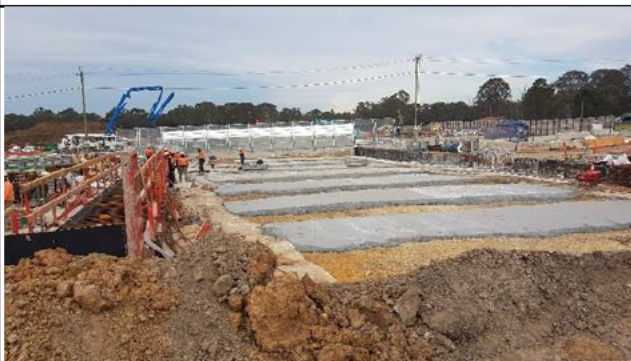
View south of Orchard Hills north of Lansdowne Rd. Capping beam FRP and blinding of girder beds.
