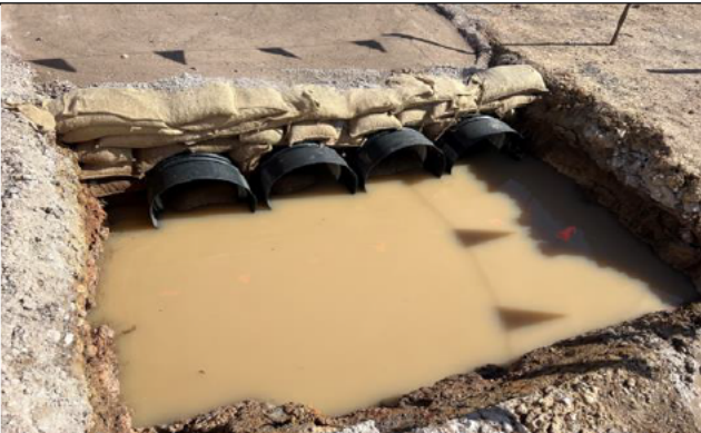
Luddenham station - Drainage directs dirty water under the haul road to a treatment location
