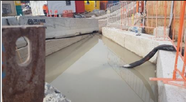
St Marys: Sump and pump installed on Station St at Gidley St (haul road), collects water off both
