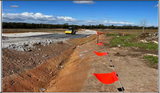
Luddenham south – Scour noted in V-drains, so need reshaping and rock checks
