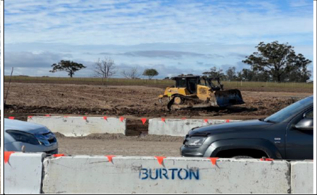
Luddenham station - Fill continues to be placed ahead of being topsoiled and hydromulched
