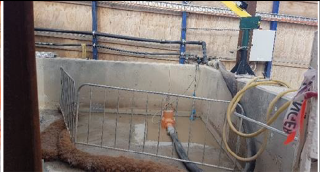
Sump and pump system installed at nib wall in the southwest corner of St Marys main laydown
