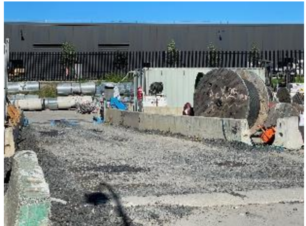
Plate 37 – Wash bay at Gate S2
