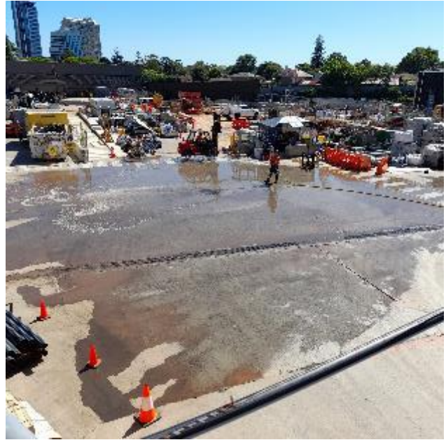
Plate 6 – Evidence of dust suppression by water spraying post the audit inspection at Chatswood Dive
