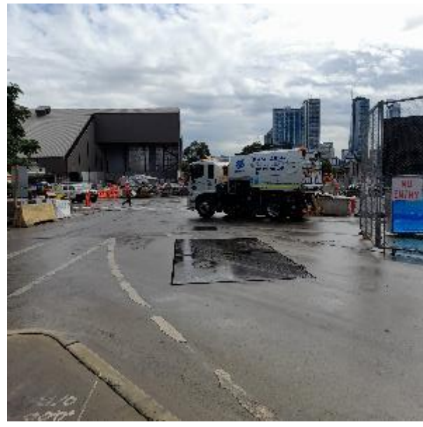
Plate 4 – Example of use of water cart and sweeper for dust suppression at Chatswood Dive
