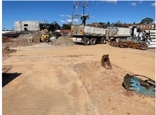
Plate 8 – Work area with exposed earth/soil and source of dust during windy conditions at the time of the audit inspection
