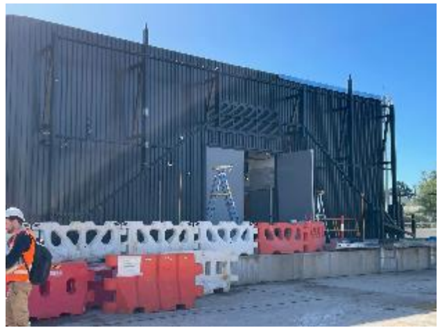
Plate 2 – Dive site service building – civil and M&E works
