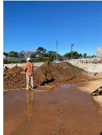
Plate 2 – Water spraying for dust suppression on hardstand and stockpiles post audit inspection at Chatswood Dive
