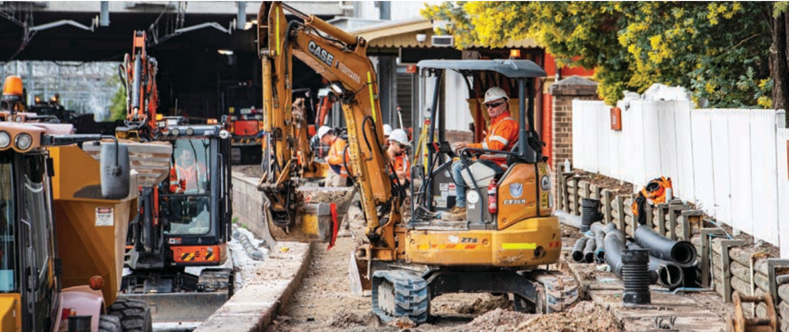
Excavation being undertaken on existing platforms at Campsie Station as part of platform reconstruction work.
