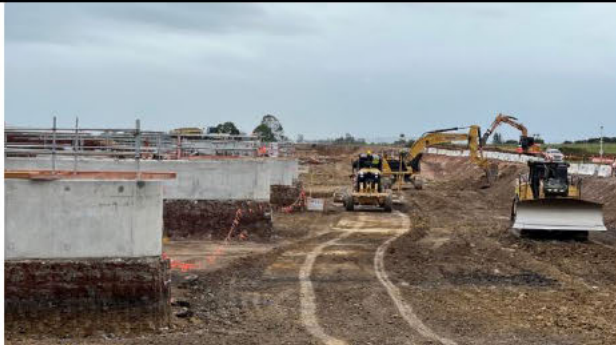
Piling pad - Excavation continues around the headstocks to allow the set up of the 500t crane and super-T delivery
