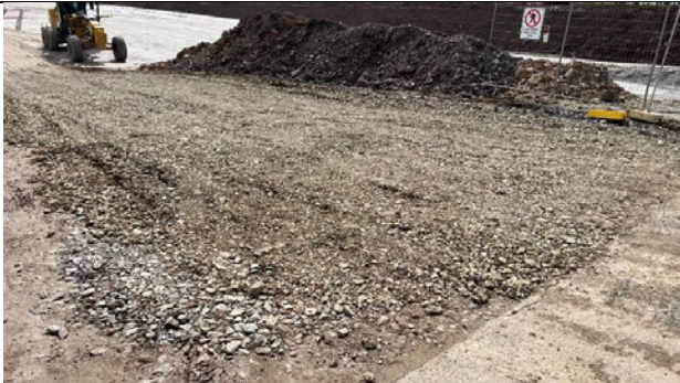
Luddenham Station - The ballast at the exit point had become full of sediment which could be tracked onto public roads
