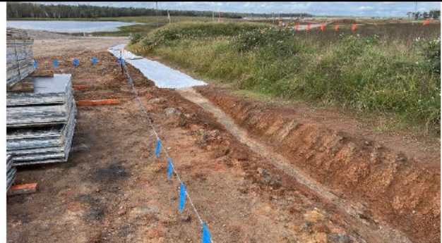
Piling pad - Geofabric and check dams have been placed in the drainage line from the piling pad
