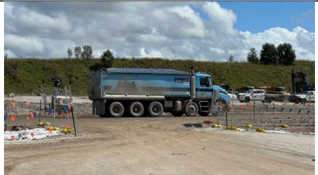
Patons Lane - Trucks from SBT are bringing material to be stockpiled at the SMF
