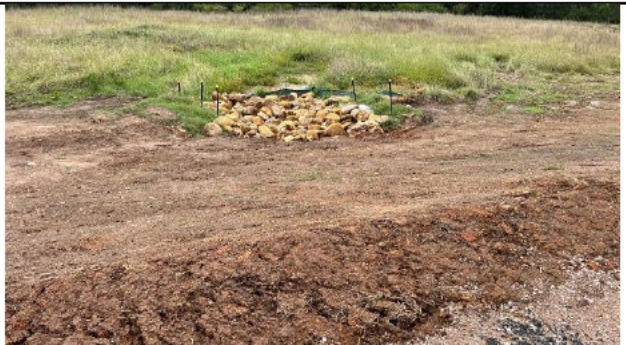
Compound access road - Site won rock is being used in erosion and sediment controls on site instead of being disposed off site
