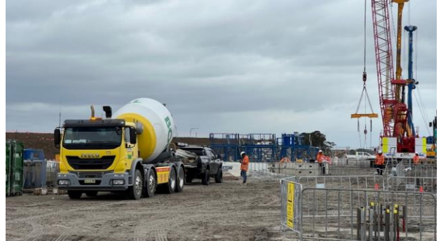
Luddenham station - All loads of concrete are being tested prior to being poured. It is noted that the trucks washout back at their depot
