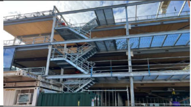
The external fire stairs are complete and fire certification works are ongoing
