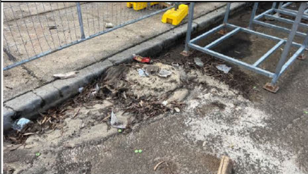
Minor amounts of rubbish at the back of the site were observed and need to be cleaned up
