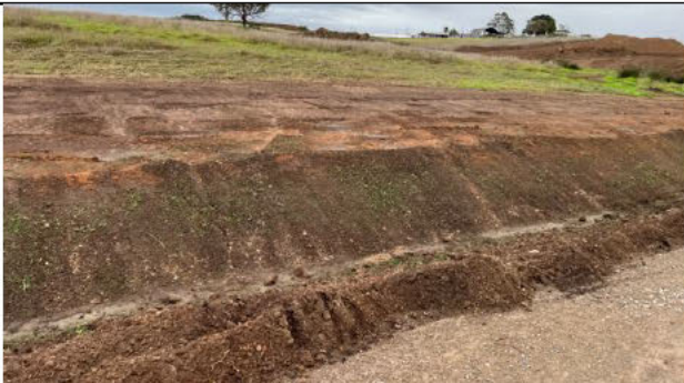
Piling pad - Green pick has started to shoot from the drainage lines and previously spread topsoil
