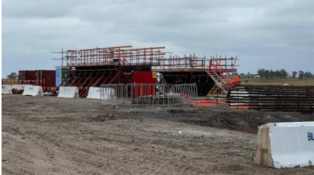
Luddenham station - Forms and reinforcement for the parapets are being constructed on site
