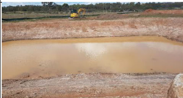
Aerotropolis view to southwest: Sed basin installed awaiting inlet pathways and spillway
