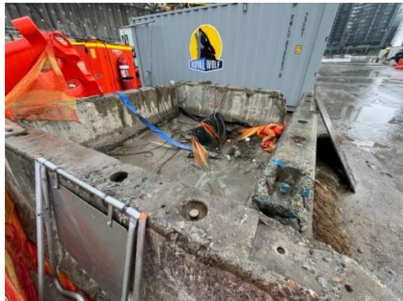
Maintenance of the surface water management system required review
