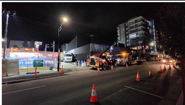
Canterbury MSB – The vacuum truck was located adjacent to the MSB, impacting the noise profile.
