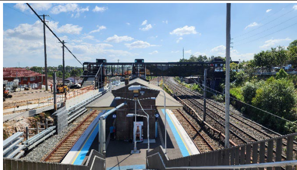
Dulwich Hill: Platforms, Plaza to the left and Footbridge stairs and roof installation in background.
