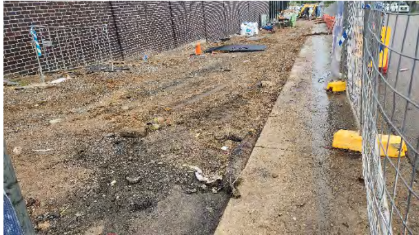
Lakemba Scouring of DGB
