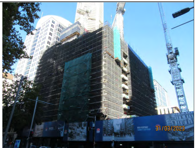
Martin Place South: Ongoing building works inside scaffolding. Ongoing use of jump form.
