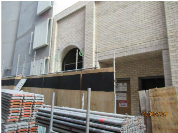
Eastern Entrance: View from Randle Lane of brick wall at rear of building.
