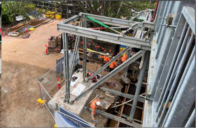
St Marys lift relocation– The temporary truss installed on the temporary pads
