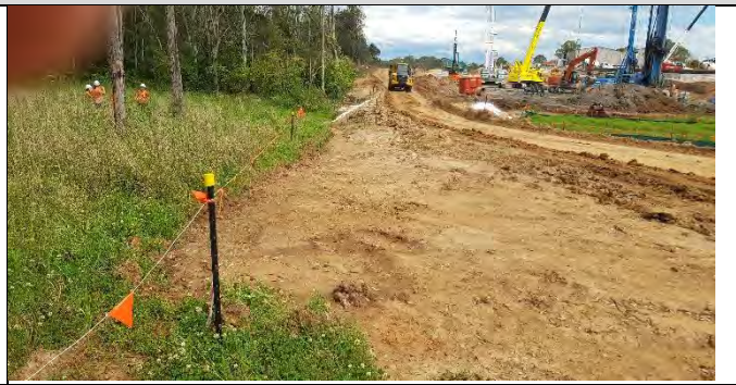
Orchard Hills north view South - ERSED controls around drainage line and crossing, require improvements
