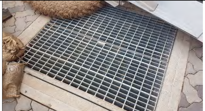
St Marys North west corner of Station St. - In path and in pit protections require improvement
