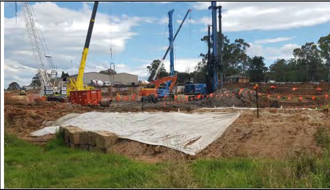
Orchard Hills north view south west: Station box and portal pilling works
