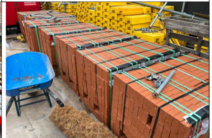
St Marys lift relocation - Additional new bricks have been procured that will supplement the reused existing bricks
