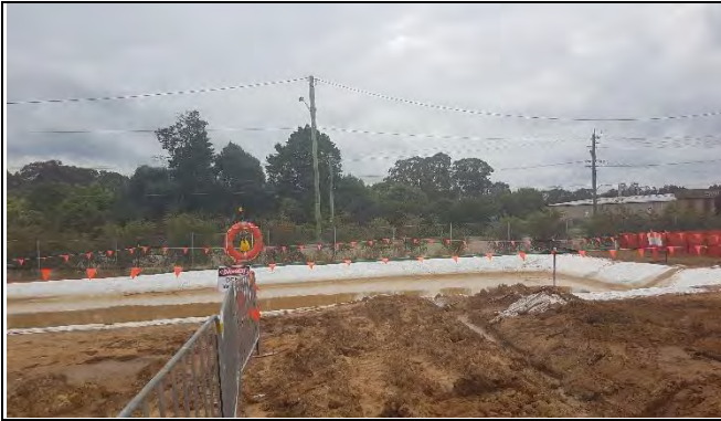
Claremont Meadows south west corner - Basins require rock and geofabric lined spillways with dissipaters.
