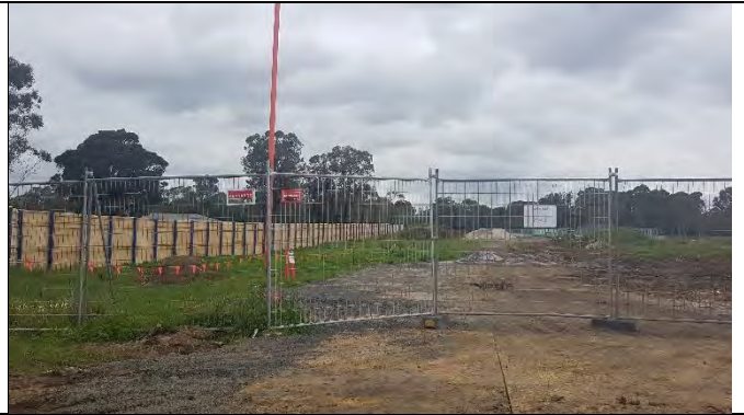
Orchard hills– South of Lansdowne Rd hoarding along west boundaries, with southern boundary remaining
