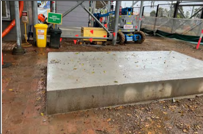
St Marys lift relocation – View of the temporary pads for the installation of the new lift shaft and removal of the old lift shaft
