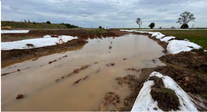
Patons Lane access to SMF view north - Controls installed retained dirty water from major rain event within the site
