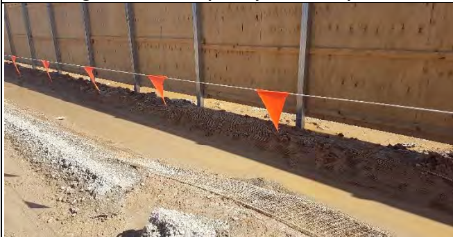
Bringelly Services Facility – Swale along Northern Boundary overflow to boundary in recent high rainfall
