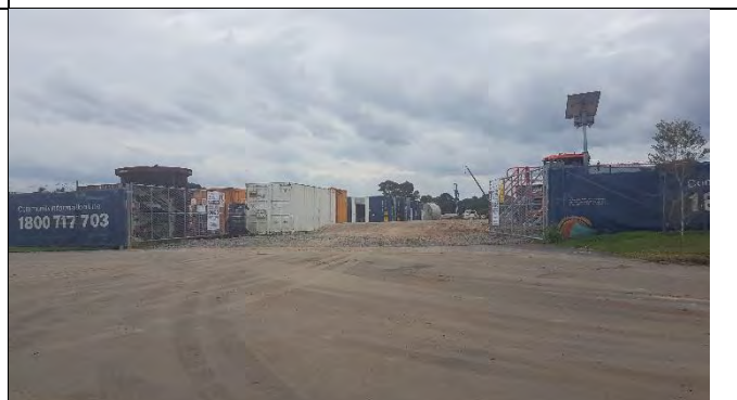
Claremont Meadows southern access - Appreciable tracking noted. CPBG to improve stabilised access
