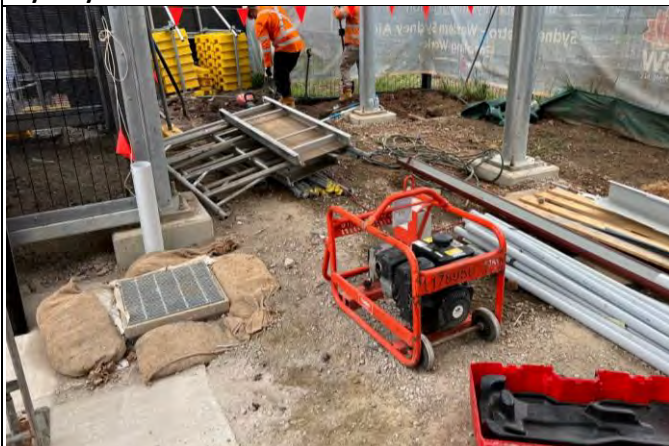
St Marys lift relocation – A small generator was observed unbundled, a bund is required during refuelling activities
