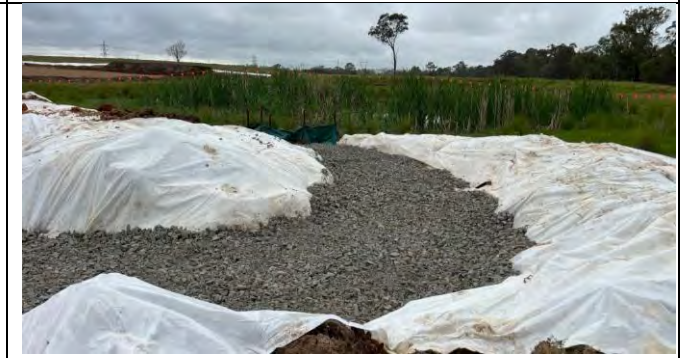
Patons Lane - A controlled drainage channel has been installed along the access road
