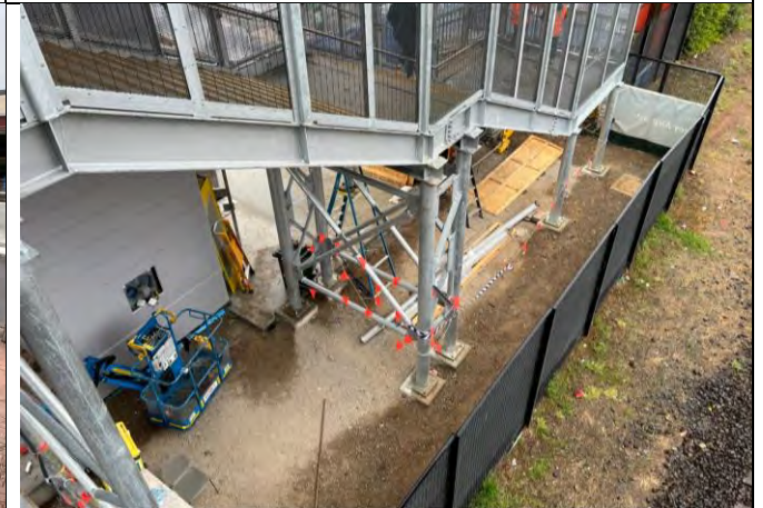
St Marys lift relocation – The site is well contained and in good order
