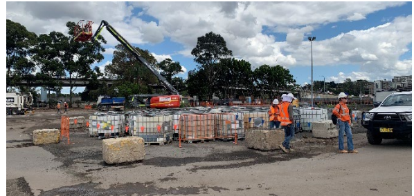
Figure 5-9: Clyde MSF chemical storage to be banded
