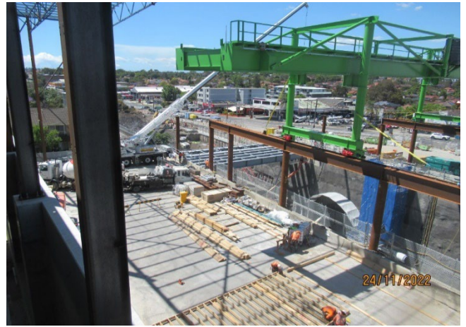
Figure 2-4 Construction of Gantry Crane and frame of the acoustic shed (Burwood North)
