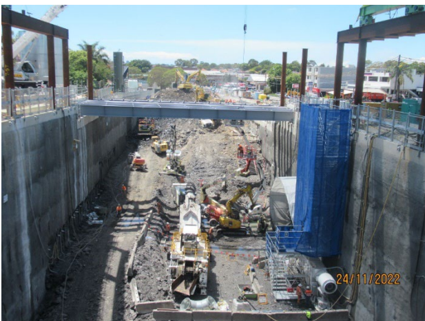
Figure 2-3 Ongoing excavation of the station box (Burwood North). Roadheader in the base of the excavation commenced tunnel excavation to the south shaft.
