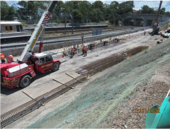
Figure 2-7 Piling on the lower side of the station box at North Strathfield
