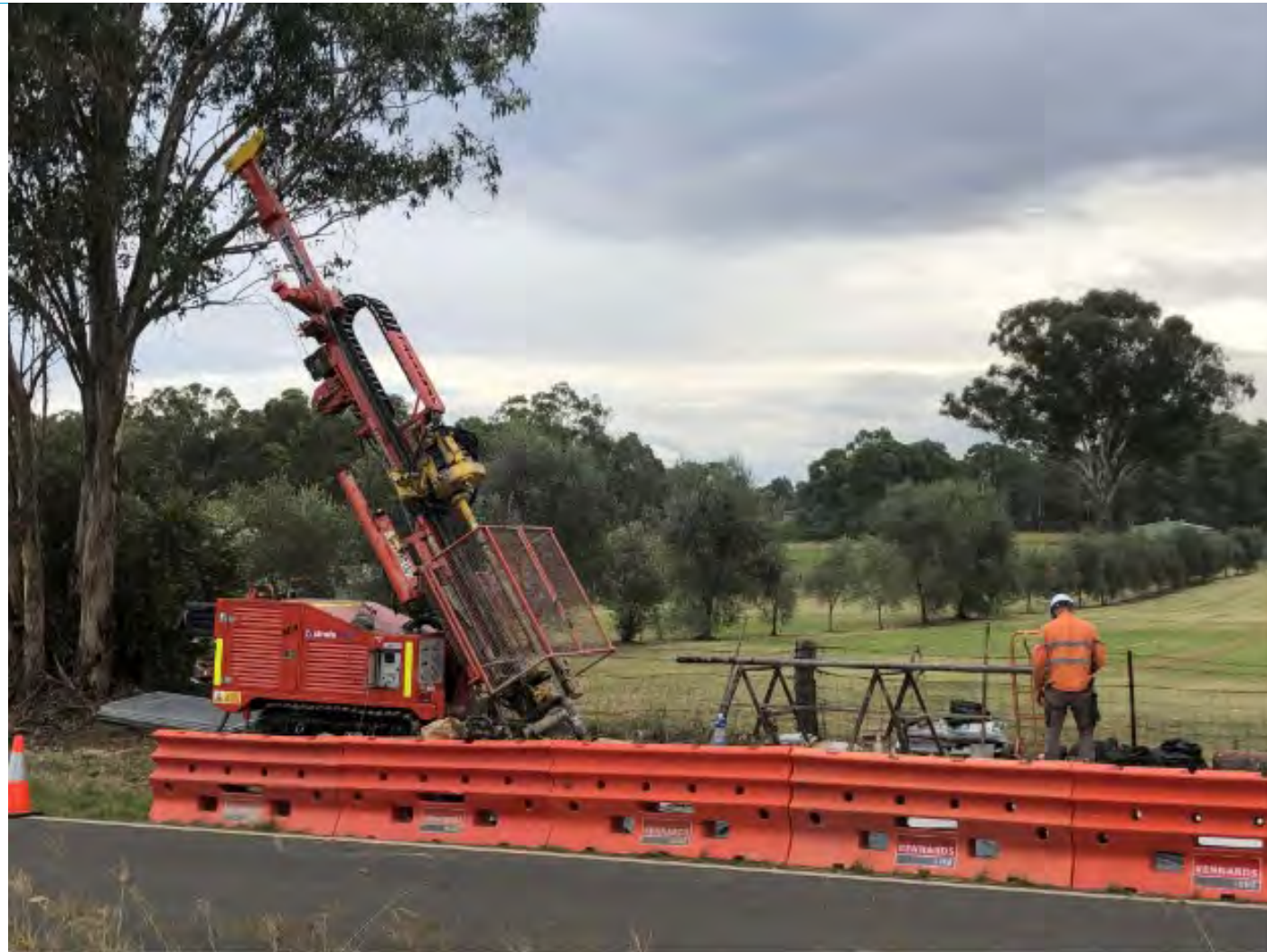
Figure 3: Example of a borehole/monitoring well set-up required for the proposed geotechnical services
