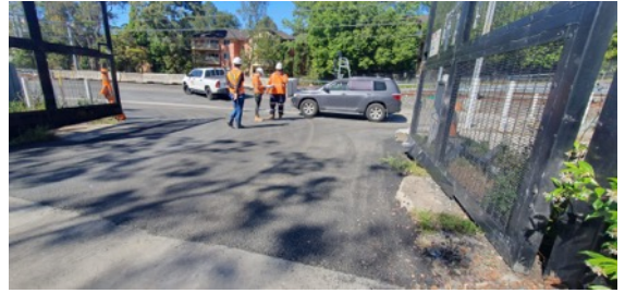
Northern Connection: Drake St – new paving installed near the site access and within the rail corridor
