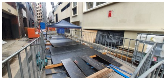
Surry Hills BPS Works - Randle Ln Joint Bay - SC reports cable installation and jointing works completed.
