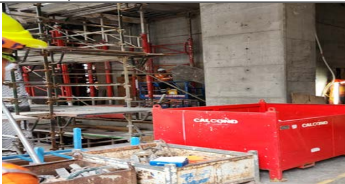
PSS Level 4 - EWP was operating using a standard movement alarm.
