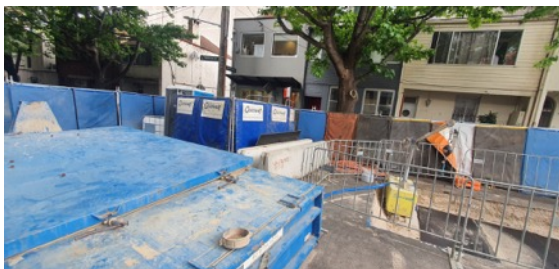
Surry Hills BPS Works – Belmore St Joint Bay: Noise blankets installed around generator (not operational at the time of inspection).
