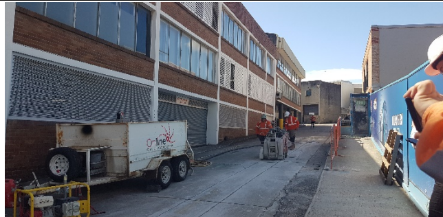
Clarke Lane South - Road Saw in use within 5 m of receivers without noise mitigation measures in place.
