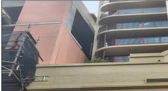
Pitt St South (PSS): Level 5 podium façade walls adjacent to Princeton Apartments.
