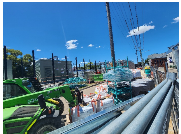
Campsie: MSB security fence poles and transformers
