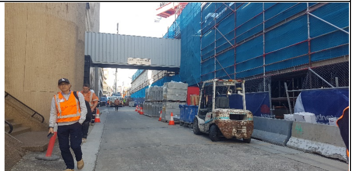
Clark Lane North – Materials and plant not stored in accordance with REMM LV1 and outside boundary.
