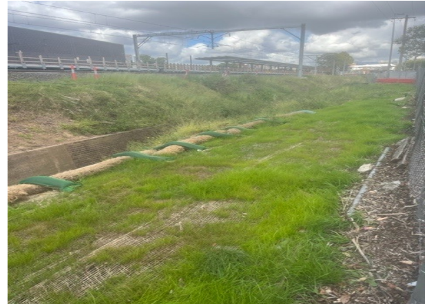
Establishment of stabilisation measures along the culvert after tree removal, Bankstown Station
