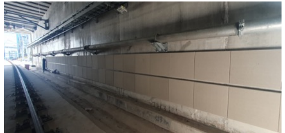
Northern Dive: Commencement of acoustic panel installation along section of Northern Dive Wall
