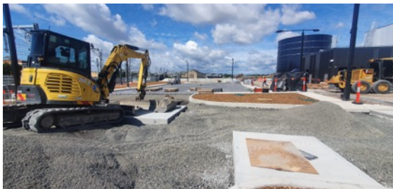
SMTF S - Future Carpark Area: Paver installation works underway for future carpark.
