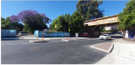
Northern Connection: Brand St drainage crossing works completed with line marking works remaining.
