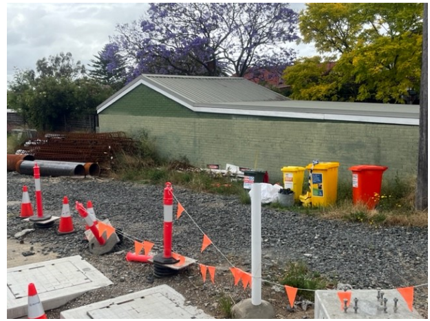
Materials stored close to private property, Melford Street Hurlstone Park
