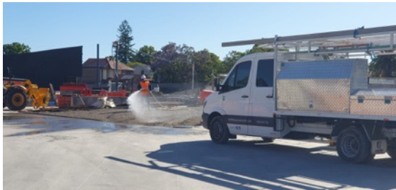
CDS - Access Ramp /Laydown Area: Dust suppression observed on access ramp and laydown area
