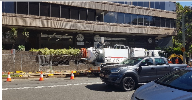
Oxley St west of Clark St – ATF fencing should include screening and information required under CoA B10.
