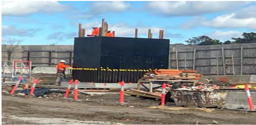
Western civil pit works commenced. Implementation of procedures for discharge of water direct to harbour to be monitored.
