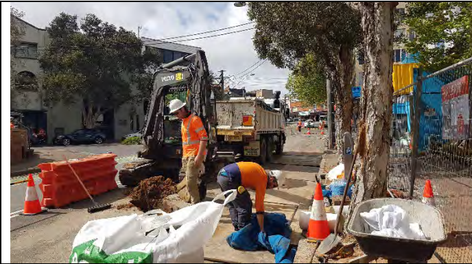
View south at Clarke St (No.28 to 30 20): Utilities works area well managed
