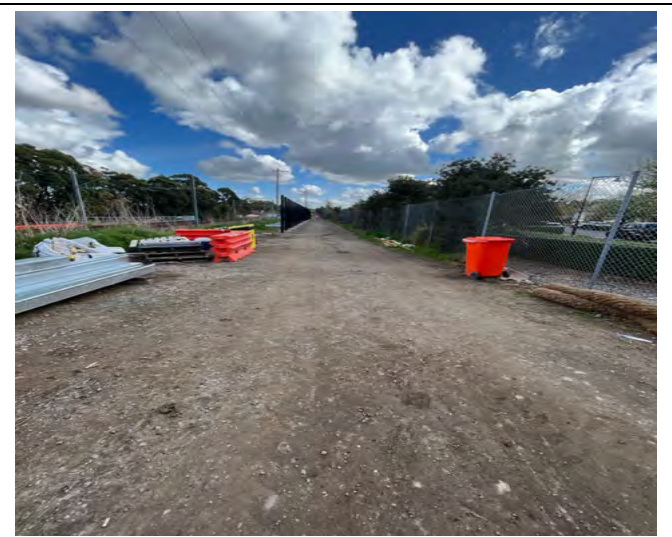
Stansfield Street, Punchbowl: Stabilised internal haul road
