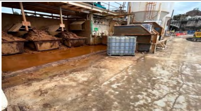
WTP and surrounds required clean up on 15/9/22
