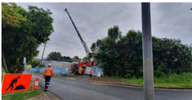
Canterbury TSS - Façade panel installation in progress with crane set-up on City End
