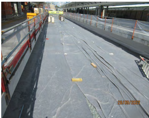
Traffic Deck: Placement of ballast on the northern section of the traffic deck completed.
