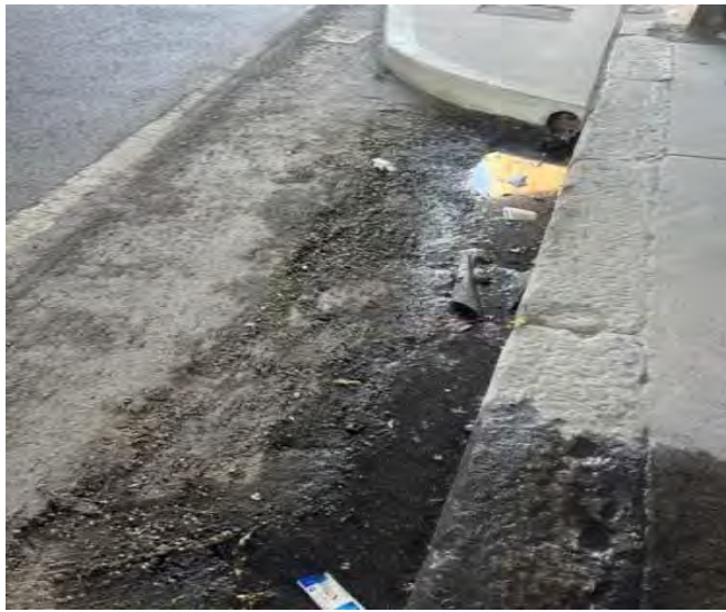
Sediment in the gutter on Hickson Road
