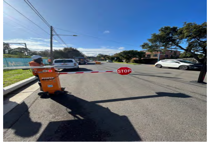
Wairoa Street Bridge, Campsie: Traffic control in place for lane closure for concrete pours
