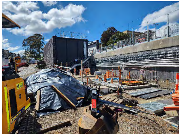
Lakemba – MSB and transformer / chiller slabs.
