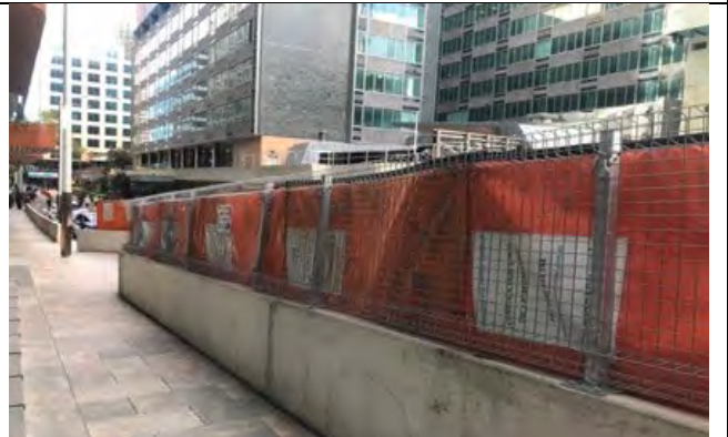
Denison St: Stage 3 stormwater worksite with noise blankets installed along section of worksite.
