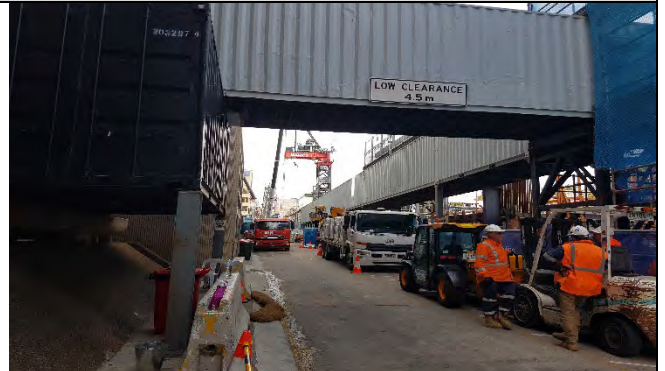
Clarke Lane North MAF – Deliveries at extended boundary encroaching on access to 26 Clarke St carpark.
