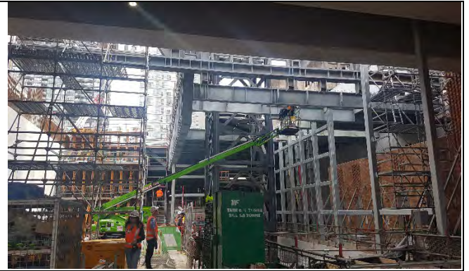
Site A - B2 to B0 concourse internal structural and slab platform steel
