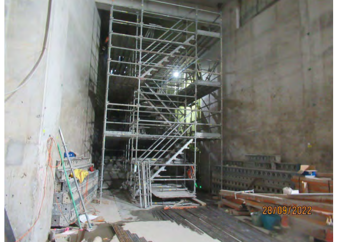
Central Walk: Completed excavation and removal of spoil from the escalator shafts at Platforms 16/17 and 18/19
