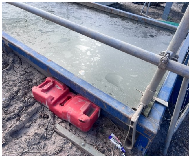
Belmore Triangle, Redman Parade: In-ground skip bin containing vacuum truck slurry was at capacity, posing risk of an uncontrolled release during the next rain event
