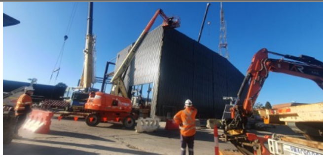
Chatswood Dive Site - Acoustic gantry shed removal underway around Northern Dive Building.
