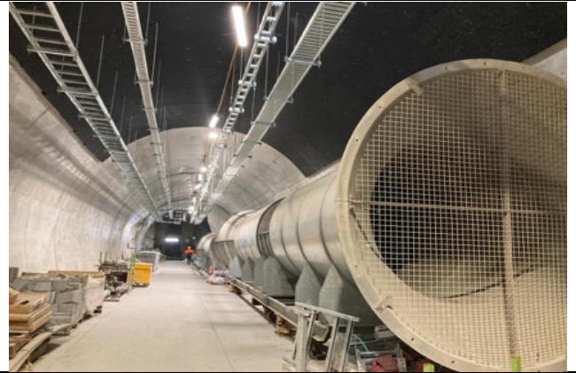
Public access to Station Cavern: Sound proofing works and cable tray installation progressing on adit roof.
