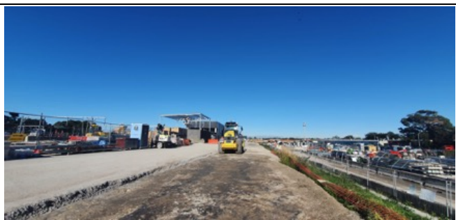
SMTF S – Stabling Yard: permanent internal access road works within SMTF S commenced.
