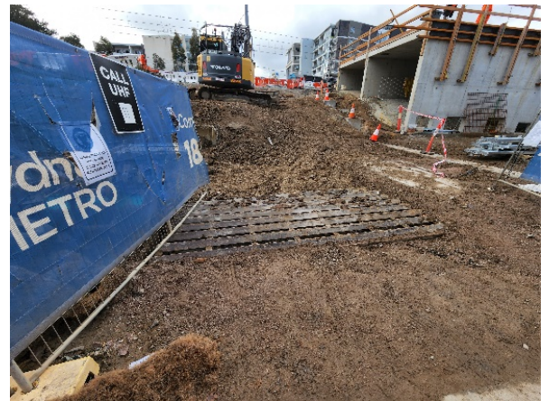
Canterbury MSB – rumble grids and egress requiring maintenance
