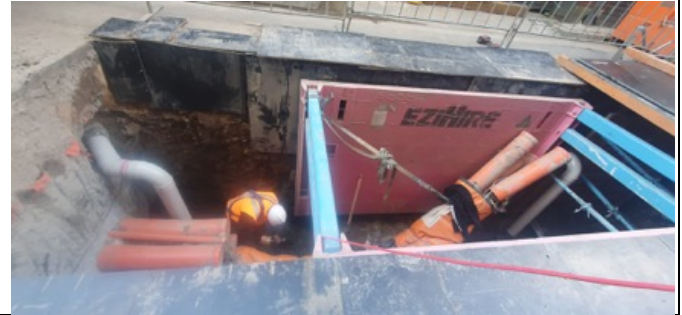
Randle Ln Joint Bay (Surry Hills): Joint bay preparation works underway for cable pulling.
