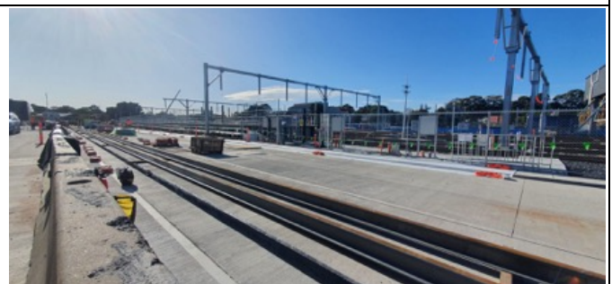
SMTF S – track slab: Rail placement and drainage preparatory works underway for track slab.
