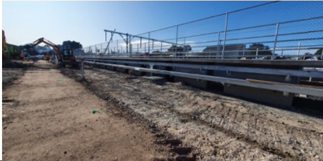
SMTF S – Platforms: Installation of fencing on platforms 7/8 and preparatory earthworks underway for swale drain.
