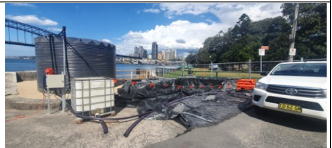
Blues Point Road – Streetscaping worksite - Tank and appropriate controls remain in place to manage and contain dirty water.
