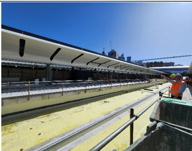
Traffic Deck: Water proofing of the northern section of the traffic deck completed.
