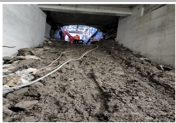
Central Walk: Ongoing excavation and removal of spoil from the escalator shafts at Platforms 16/17 and 18/19
