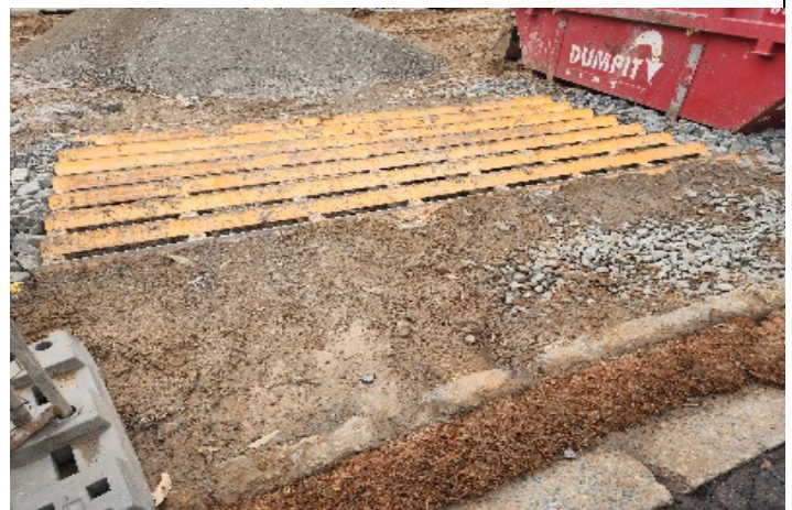
Hurlstone Park: MSB storage of bins outside boundary, MSB egress requiring maintenance
