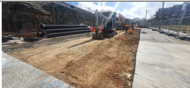
Blues Point Road – Streetscaping worksite – Preparatory works for load out of subgrade material from worksite underway.
