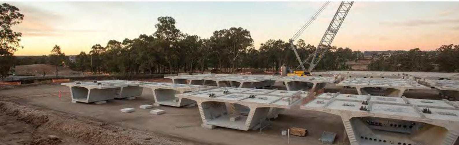
Concrete segments in holding yard on the Metro North West project. Similar segments will be manufactured for the Sydney Metro – Western Sydney Airport project at the Precast Facility in Buchanan.
