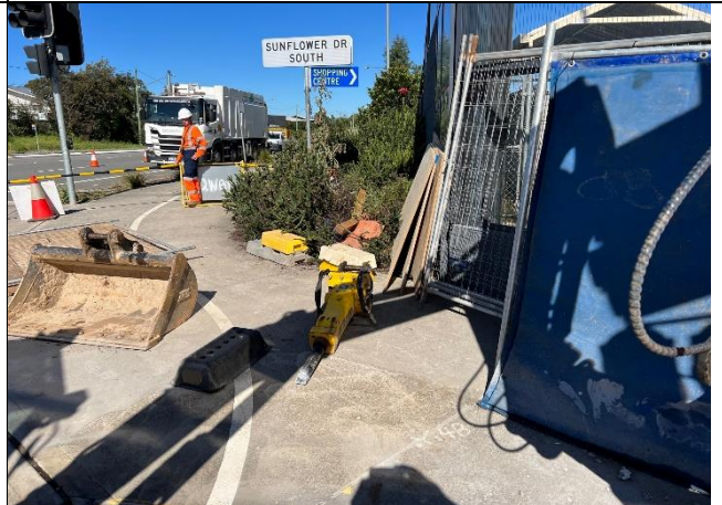
Power – Sunflower Dr. equipment placed on vegetation
