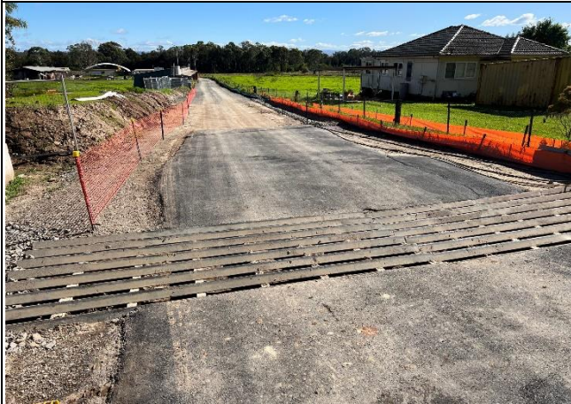
Power –Lawson Road compound entrance
