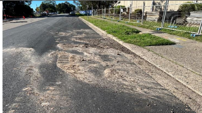
TBI entrance Station St – Clay and millings was observed.
